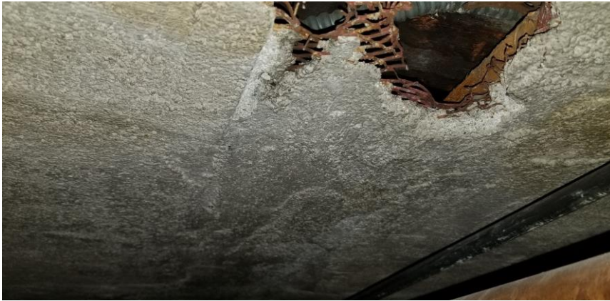
Photo 1: View of asbestos-containing plaster applied on to steel mesh observed to be in poor condition on the ceiling of the basement level boiler room.
