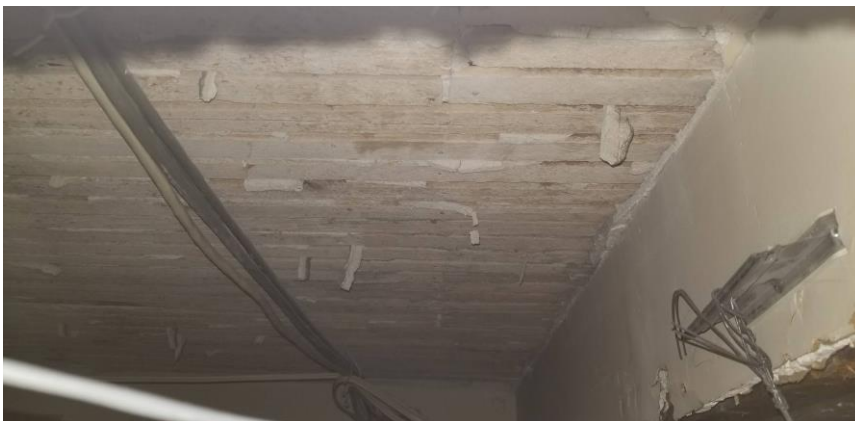
Photo 3: View of non-asbestos containing plaster on wood lathe observed above the suspended ceiling tiles in Room 204.
