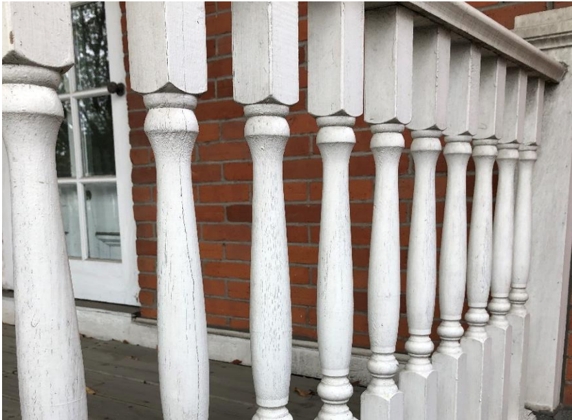
Photo 12: View of low-level lead paint (white) observed to be in poor condition on the exterior balcony/porch.
