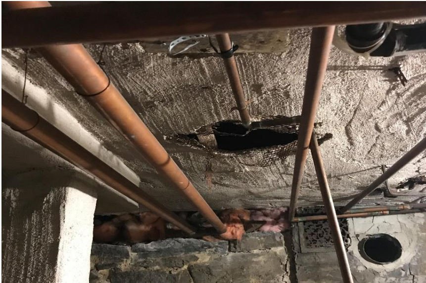
Photo 10: View of asbestos-containing textured plaster observed on the basement ceiling.
