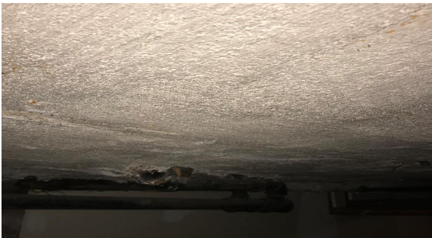
Photo 9: View of asbestos-containing textured plaster observed on the basement ceiling.
