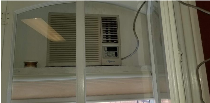
Photo 7: View of ODS-containing air condition unit observed to be in good condition in Room 204.
