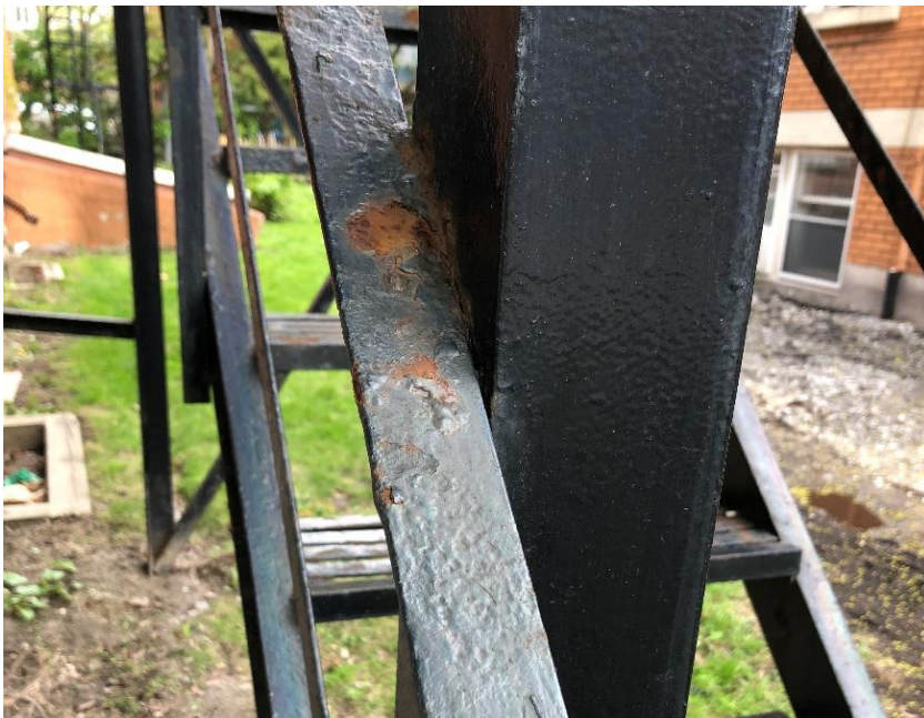
Photo 13: View of low-level lead paint (black) observed to be in poor condition on the exterior fire escapes
