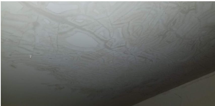
Photo 8: View of water-stained ceiling plaster observed to be in poor condition above the suspended ceiling tiles in Room 202.
