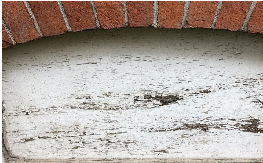
Photo 11: View of low-level lead paint (white) observed to be in poor condition on the exterior of the building.
