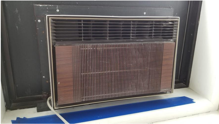
Photo 13: View of Electrohome-brand air conditioning unit observed to be in good condition in Room 216.
