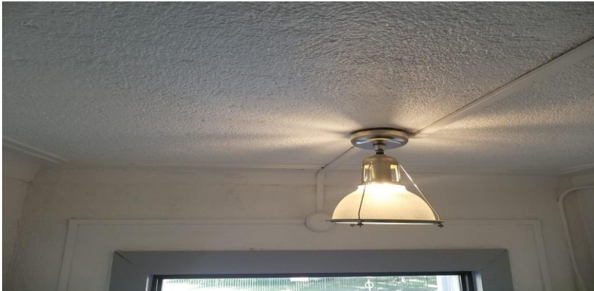
Photo 7: View of asbestos-containing ceiling texture coat observed to be in good condition adjacent to Rooms 120 and 120A.
