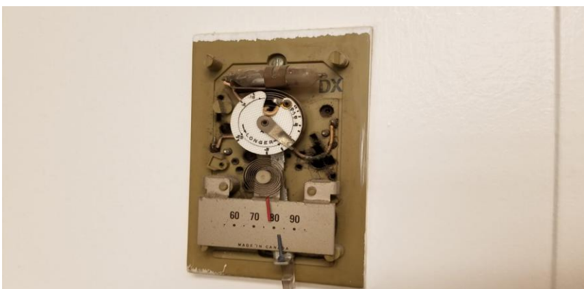
Photo 12: View of Honeywell thermostat containing one ampoule of liquid mercury observed to be in good condition in Room 013.
