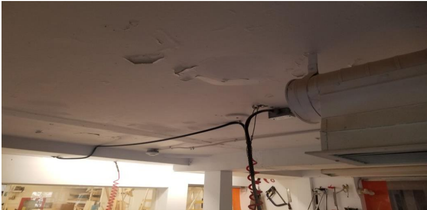
Photo 10: View of lead-containing white ceiling paint observed to be in poor condition in Room 100C.
