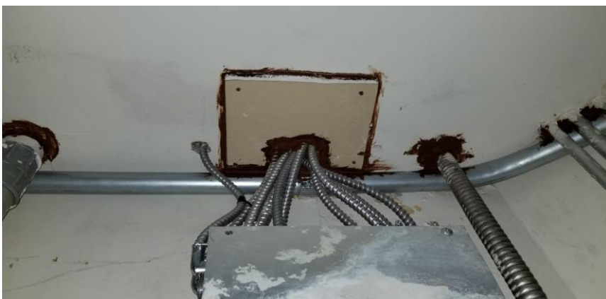
Photo 6: View of asbestos-containing firestop caulking (Red) observed to be in good condition in Room 105.
