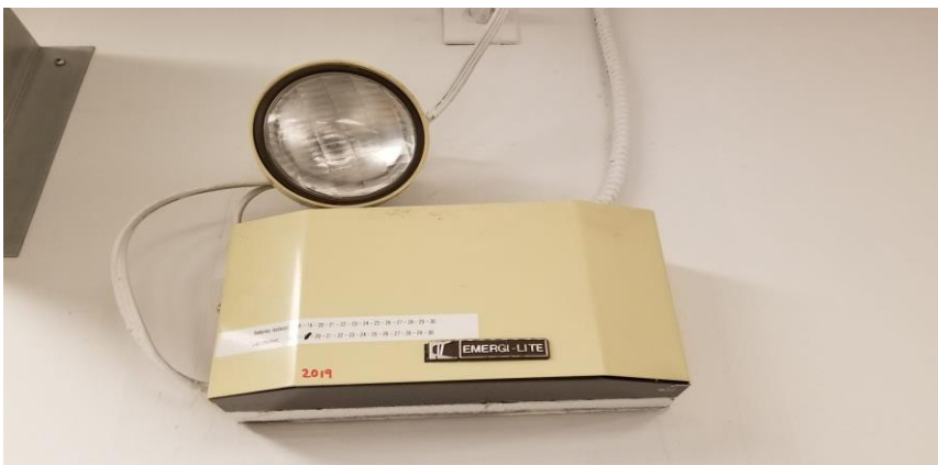
Photo 11: Typical view of lead-containing emergency battery packs observed to be in good condition throughout the surveyed building.
