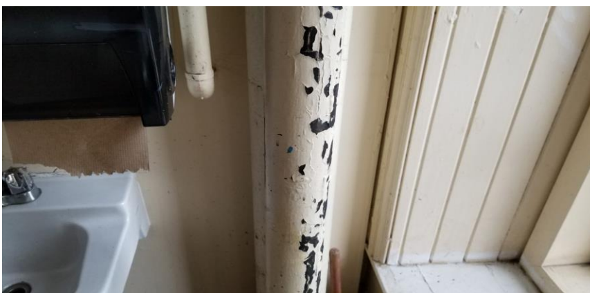
Photo 9: View of lead-containing beige paint observed to be in poor condition in Room 316A.
