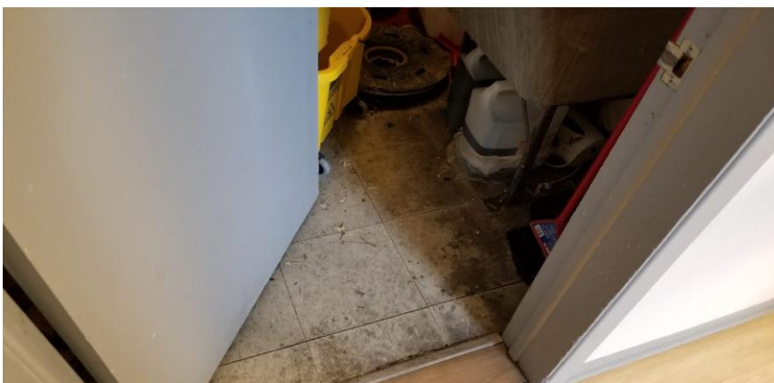
Photo 3: View of asbestos-containing vinyl floor tiles (12"x12"- Beige w/ Brown Flakes) observed to be in poor condition in Room 314. Removed September, 2020.
