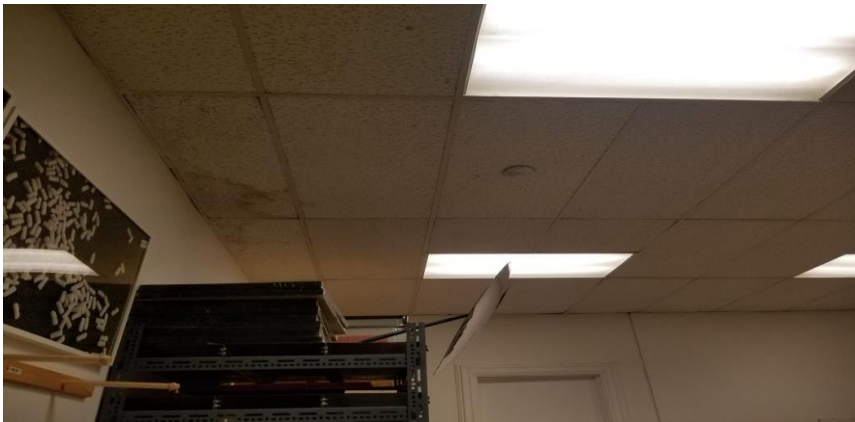
Photo 14: View of water-stained ceiling tiles observed in Room 113. Removed Summer, 2022.
