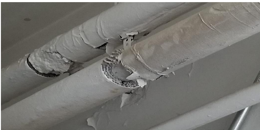
Photo 8: View of asbestos-containing pipe straight aircell insulation observed to be in poor condition in Room 010. Repaired September 2020.
