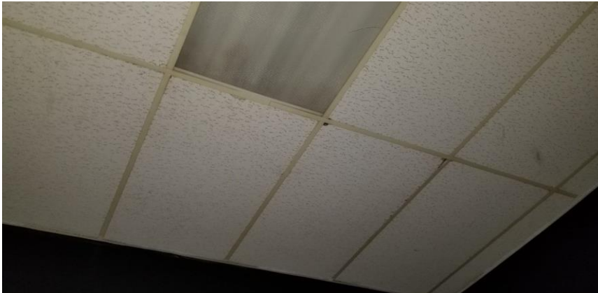
Photo 1: View of asbestos-containing ceiling tiles (2'x4'-Large fissures with pinholes) observed to be in fair condition in Room 321. Removed Summer, 2022.
