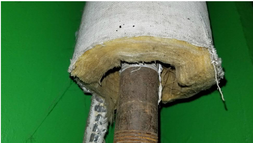
Photo 11: Representative view of the non-asbestos pipe straight insulation observed throughout the subject building.
