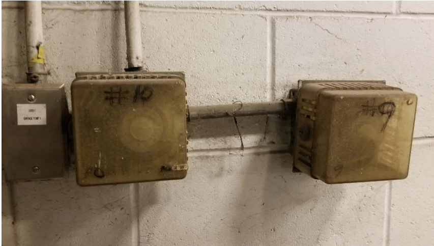
Photo 13: Representative view of the mercury-containing thermostat switches identified in Room 019.
