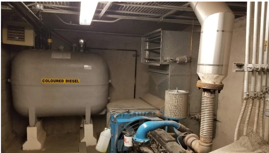
Photo 5: View of the above ground diesel storage tank identified in Room 005.
