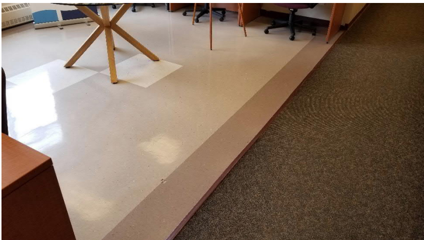
Photo 3: Representative view of the non-asbestos vinyl floor tiles and carpet mastic observed in the subject building.
