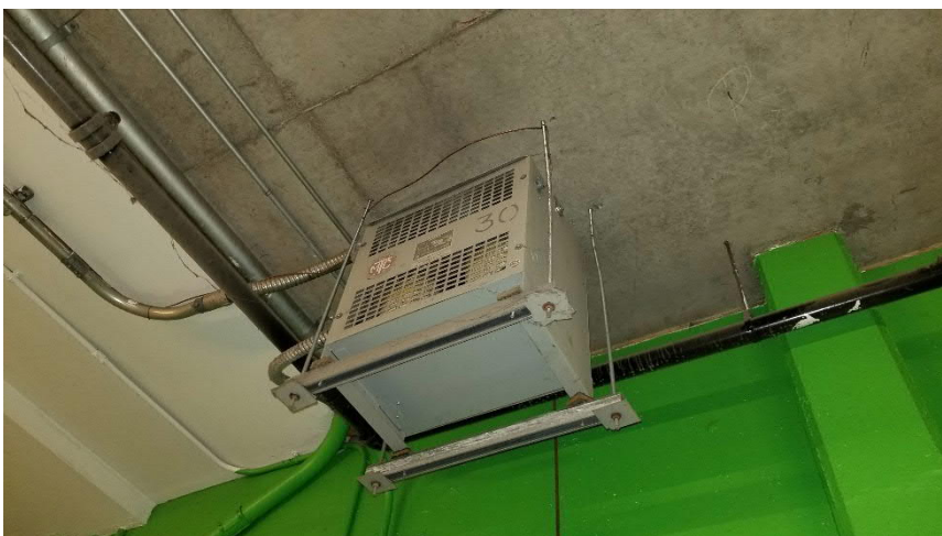
Photo 12: View of the non-PCB dry-type transformers observed throughout the subject building.
