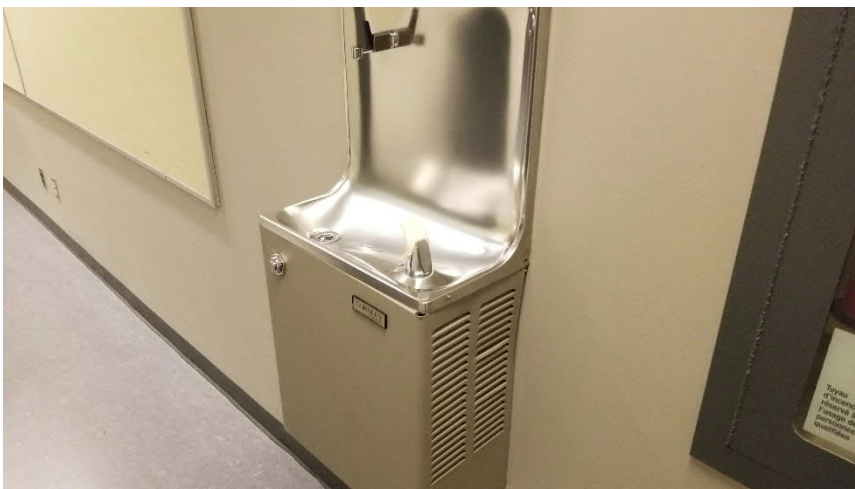
Photo 6: Representative view of the equipment containing ODSs identified throughout the subject building.
