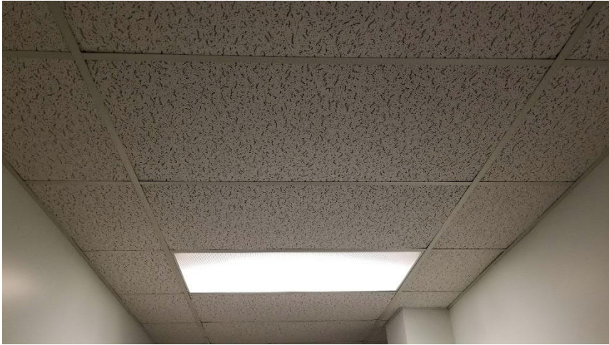
Photo 4: Representative view of the non-asbestos ceiling tiles identified throughout the subject building.
