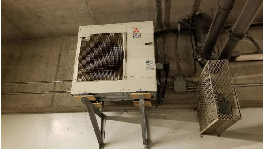
Photo 10: Representative view of the ODS containing air conditioning units observed throughout the subject building.
