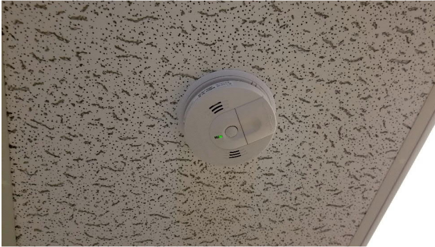
Photo 7: Representative view of the smoke detectors containing radioactive materials observed in the subject building.
