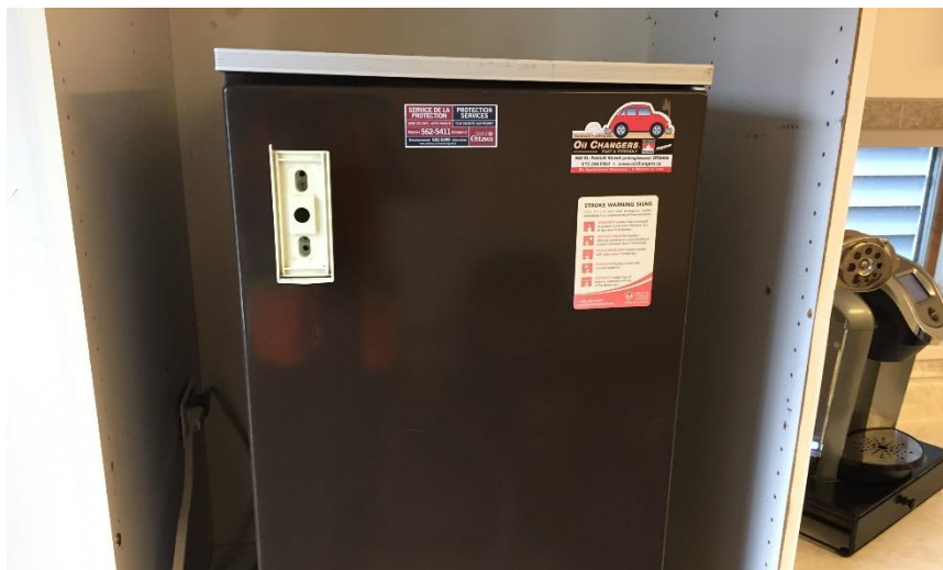
Photo 4: View of the ODS-containing equipment observed in the subject building.
