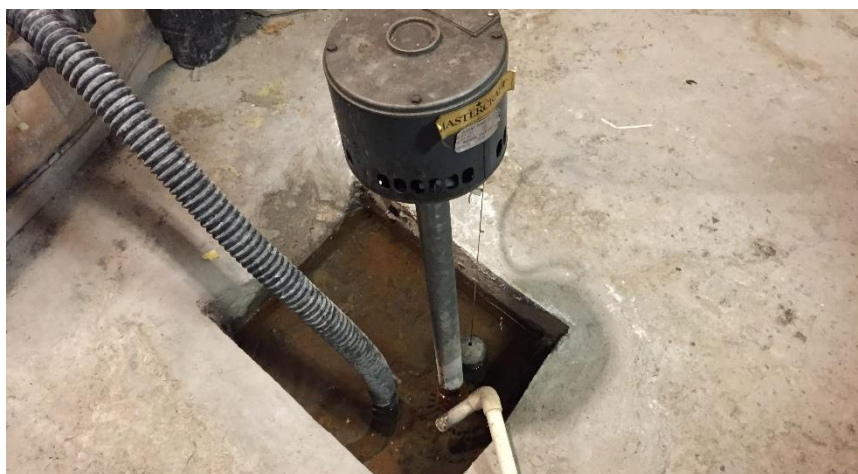
Photo 5: View of the sump pump containing a mercury float switch observed in Room B1.
