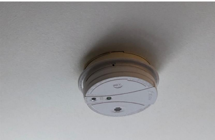
Photo 3: Typical view of smoke detectors containing radioactive materials.
