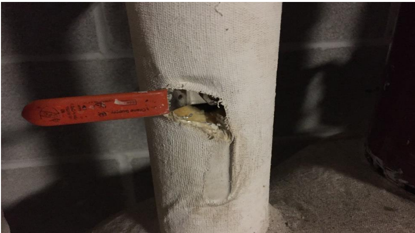
Photo 5: Typical view of fibreglass mechanical insulation.
