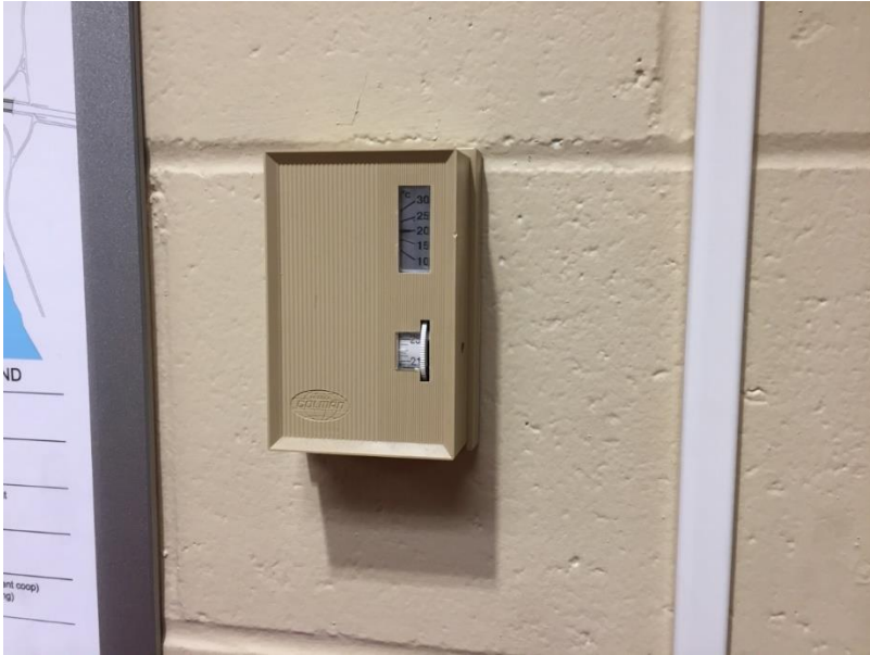
Photo 9 View of Thermostat suspected to contain mercury in Room 120A
