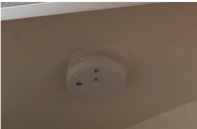
Photo 6: View of radioactive containing smoke detector observed in Room 300.
