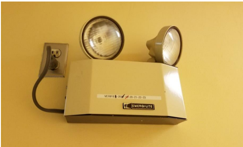
Photo 5: Typical view of lead-battery packs observed throughout the subject building.
