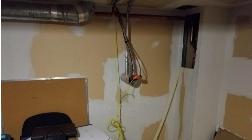
Photo 1: Typical view of asbestos-containing drywall joint compound observed throughout the subject building.
