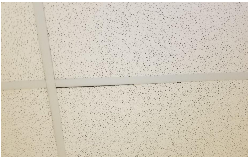
Photo 3: Typical view of non-asbestos-containing suspended ceiling tiles observed throughout the subject building.
