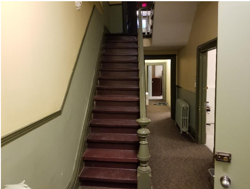
Photo 4: View of the vinyl sheet flooring over stairs with beige, light green and dark green lead paints identified throughout the subject building.
