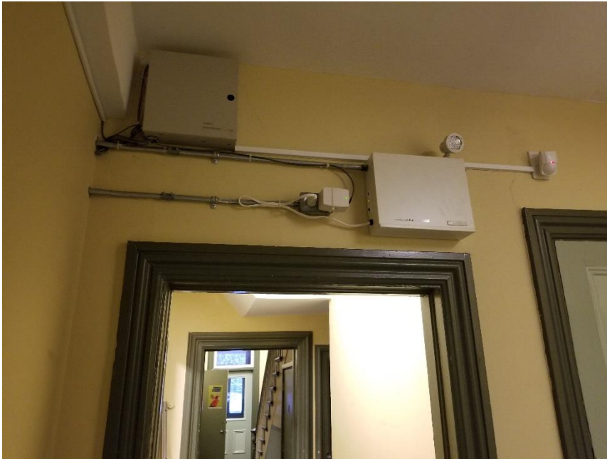
Photo 11: Emergency lighting present throughout the subject building. Lights are expected to contain lead-acid batteries
