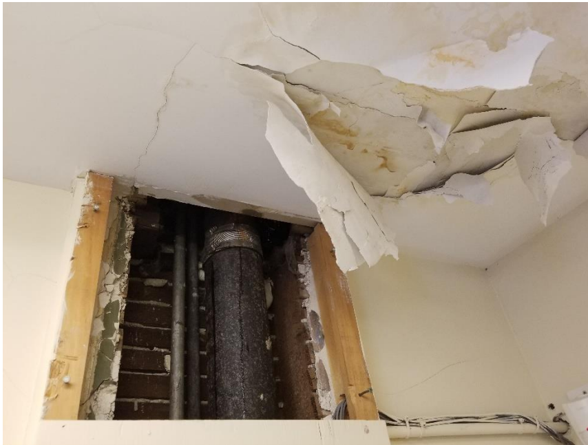
Photo 9: View of the poor condition asbestos-containing drywall joint compound peeling on ceiling from apparent water damage.
