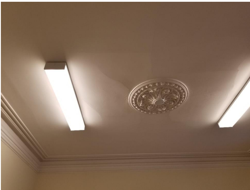
Photo 12: Typical view of florescent tube lights containing mercury vapour.
