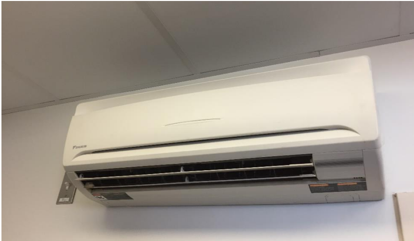
Photo 4: View of the equipment containing ODSs observed throughout the subject building.
