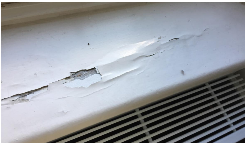
Photo 5: View of the poor condition lead paint (White) observed in Room 303.
