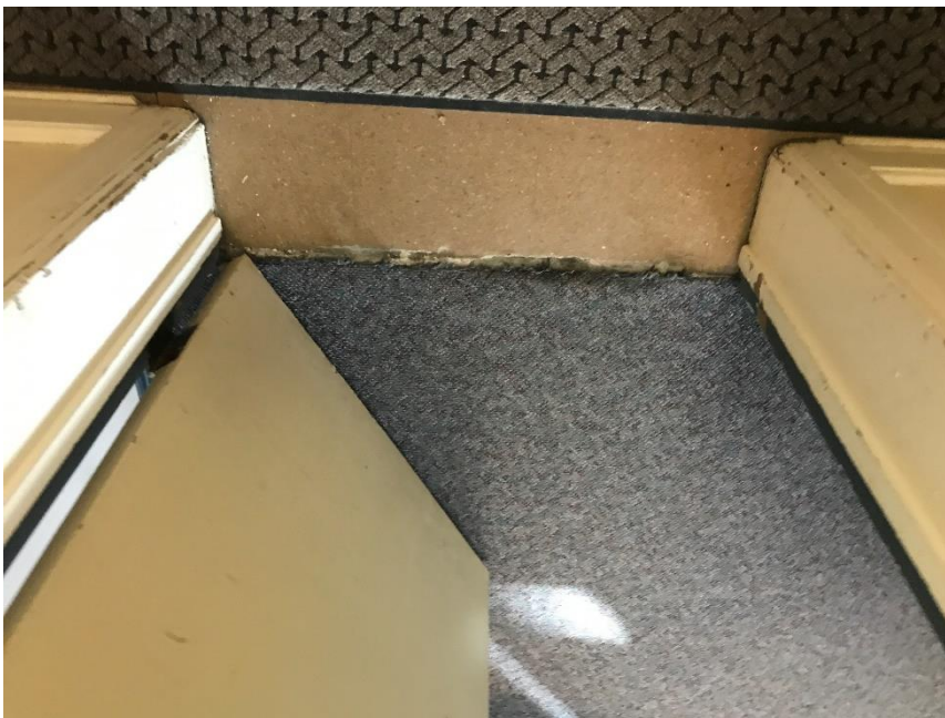
Photo 2: View of asbestos-containing vinyl sheet flooring (grey) underneath the carpet observed in Room 223.
