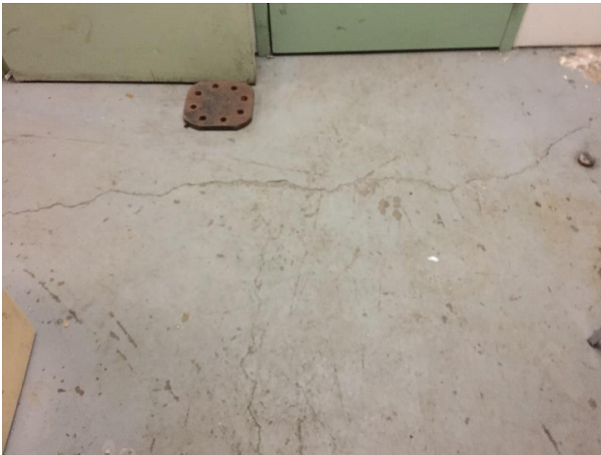
Photo 4: View of low level lead-containing grey paint within Room 06A observed to be in good condition.
