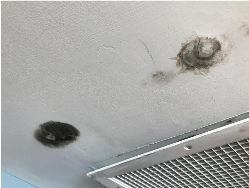
Photo 7: View of mould on ceiling in Room 229
