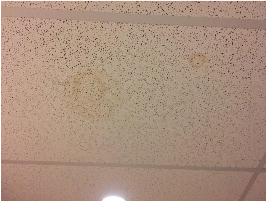
Photo 3: View of water damaged suspended ceiling tiles observed in Room 100.
