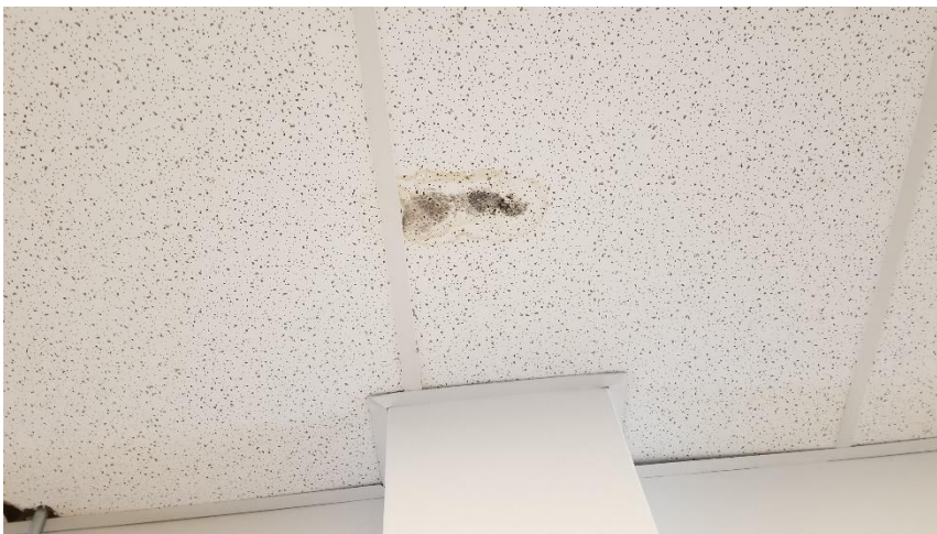
Photo 24: View of the mould impacted ceiling tile observed in Room 100.
