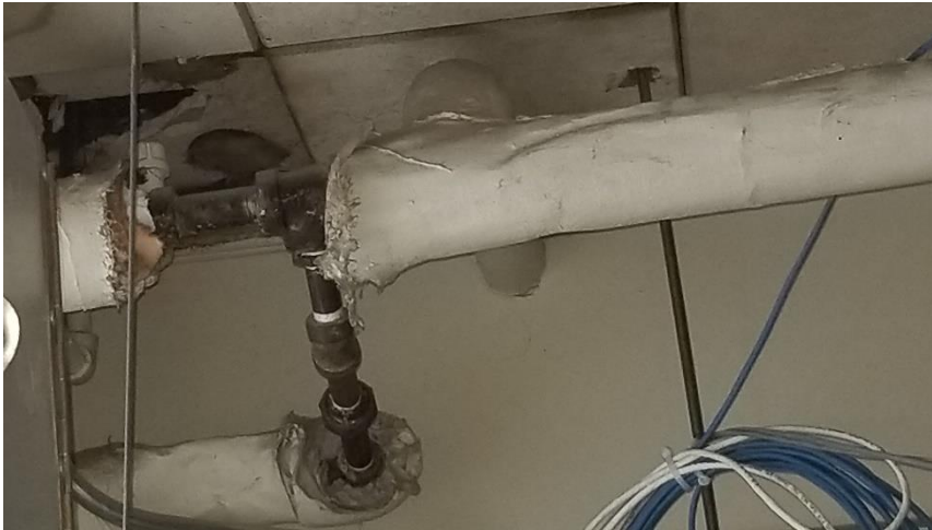
Photo 13: Poor condition asbestos-containing paring cement elbows were observed in Room 010, above suspended ceiling tiles.
