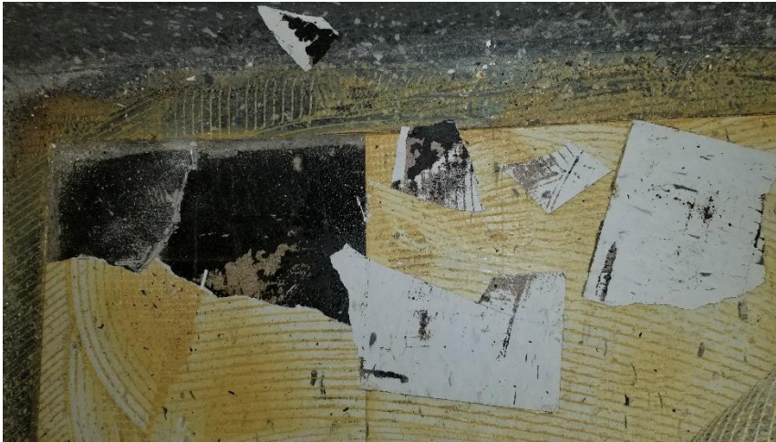
Photo 22: View of asbestos-containing vinyl floor tile mastic (Black) observed to be in good condition on the underside of the carpet in Room 07.
