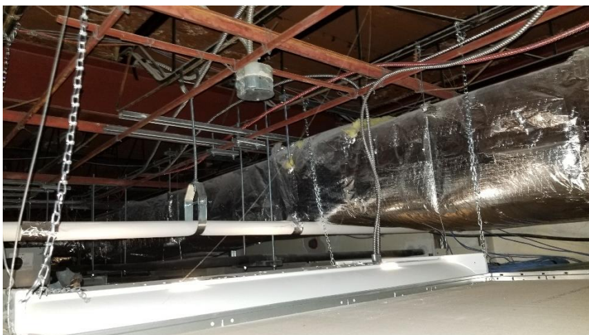
Photo 9: Representative view of the ceiling space throughout Level 1, with visible fiberglass mechanical insulation throughout.
