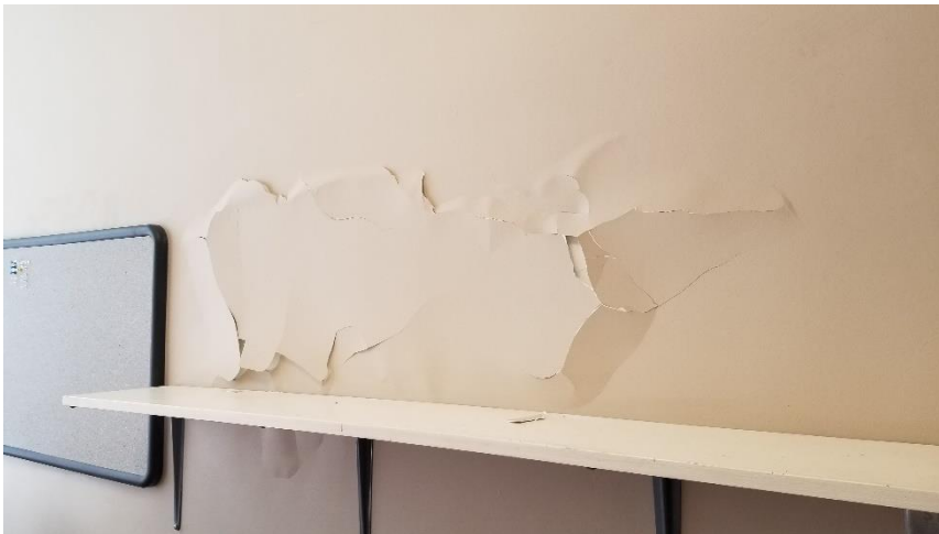
Photo 5: View of the Beige low-level lead wall paint observed in poor condition in Room 111.
