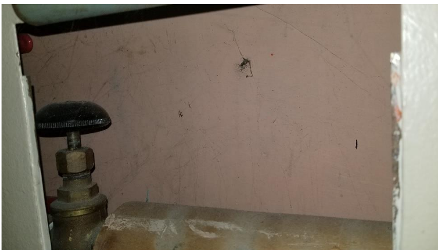
Photo 21: View of the Light Pink paint observed in Room 012, which was determined to contain low levels of lead, and enclosed behind radiator units.
