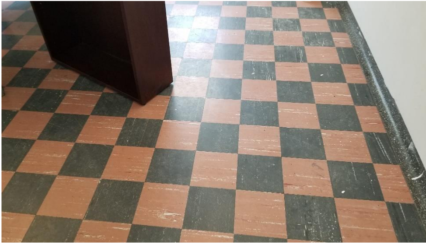
Photo 4: View of the asbestos-containing VFT 9"x9" - Pink & Dark Grey observed in good condition in Room 114B.
