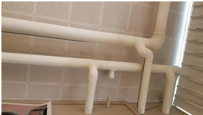
Photo 17: Representative view of the asbestos-containing parging cement elbows observed in good condition in Room 03.
