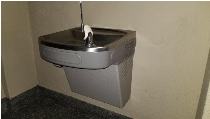
Photo 14: Representative view of the ElKay drinking water fountains observed throughout the subject building, containing a R134a refrigerant.
