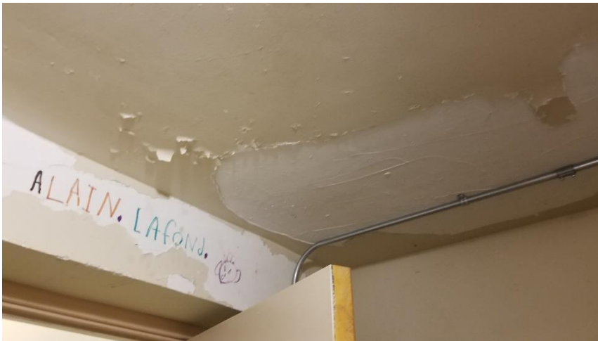
Photo 11: View of the poor condition low level lead paint (Beige) observed in Room 02A.
