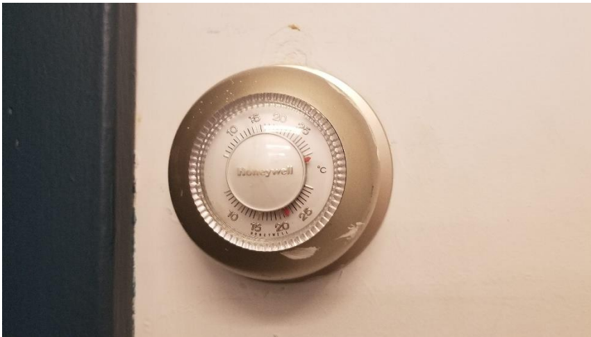
Photo 23: View of Honeywell thermostat containing one ampoule of liquid mercury observed to be in good condition on Room 07.
