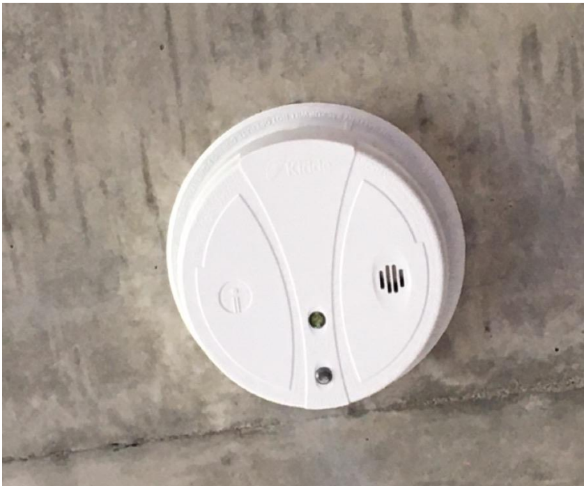
Photo 2: Typical view of smoke detectors containing radioactive materials observed throughout the subject building.
