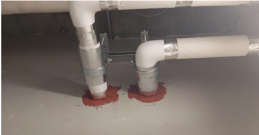
Photo 7: View of the non-asbestos containing firestop caulking (Red) observed throughout the subject building.
