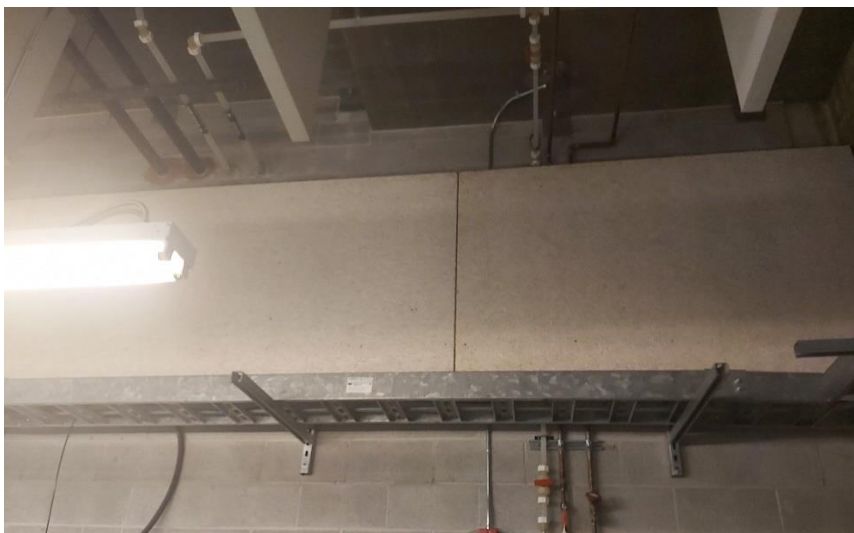
Photo 6: View of the asbestos-containing transite panels observed in Room 010.
