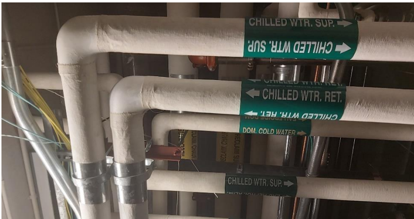
Photo 2: Representative view of the non-asbestos containing mechanical insulation observed throughout the subject building.
