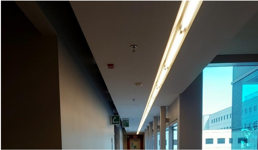
Photo 10: Representative view of the fluorescent light fixtures containing mercury vapour observed throughout the subject building.
