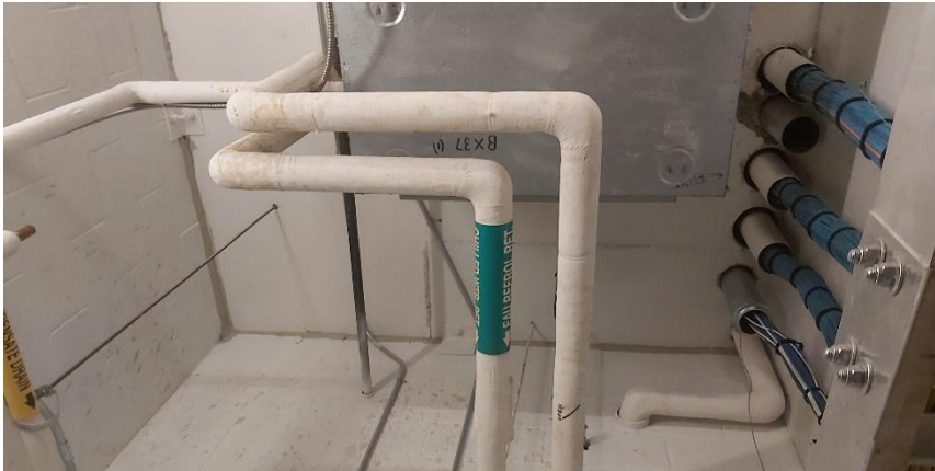
Photo 1: Representative view of the non-asbestos containing mechanical insulation observed throughout the subject building.
