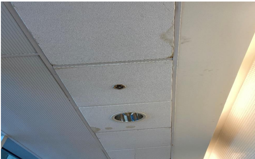
Photo 11: View of water damaged acoustic ceiling tiles (Non-ACM).
