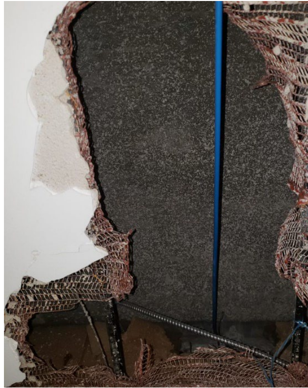
Photo 9. Example of smooth plaster in poor condition.
