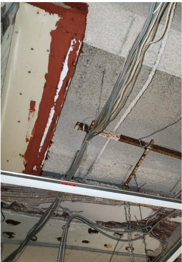
Photo 4. Example of cementitious overspray on concrete deck.
