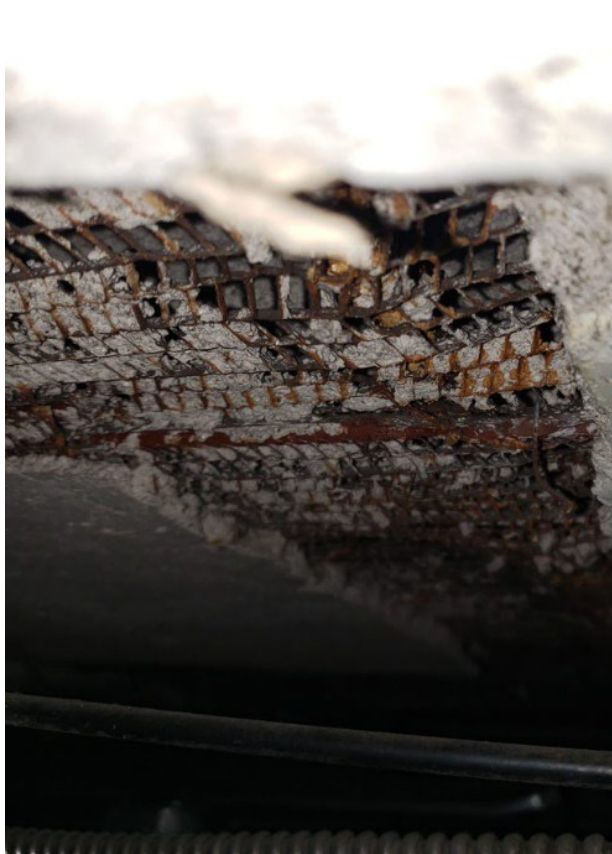
Photo 3. Example of cementitious overspray observed in poor condition.
