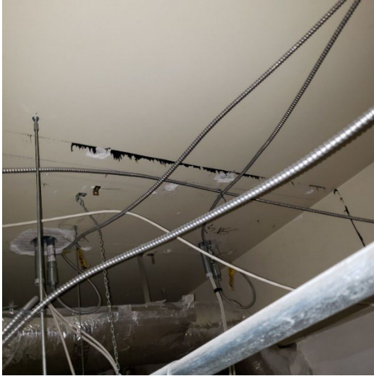
Photo 4. Example of ACM tar observed in good condition on the 1 st floor.
