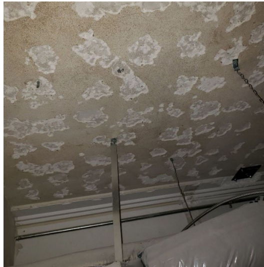
Photo 8. Example of non-ACM skim coat observed on the 4 th floor.
