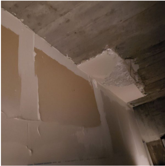
Photo 2. Smooth plaster above acoustic ceiling tiles observed in poor condition within room 5075A.
