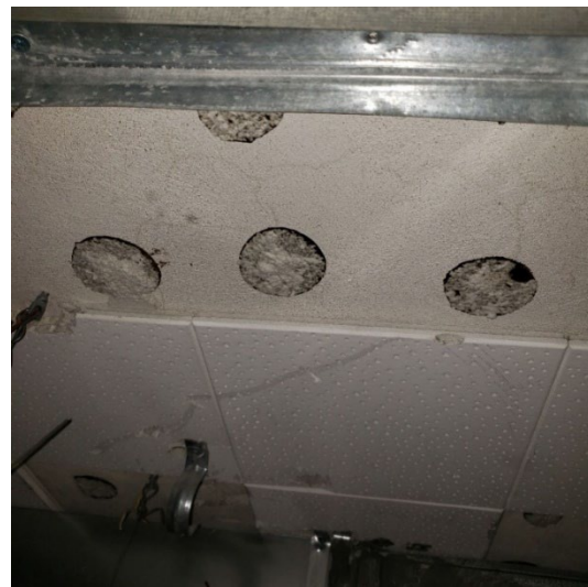
Photo 7. Example of ACM brown puck mastic observed on the 3 rd floor.
