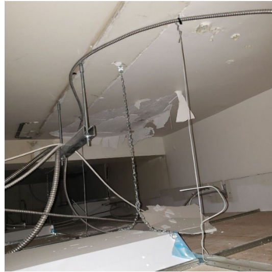
Photo 3. Smooth plaster debris observed above acoustic ceiling tiles within room 3040.
