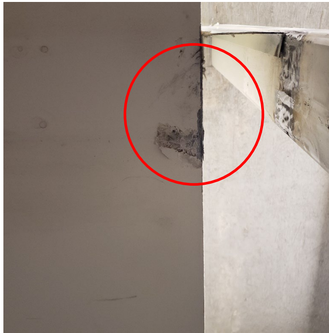
Photo 3. Smooth plaster observed in poor condition within stairwell 3C.
