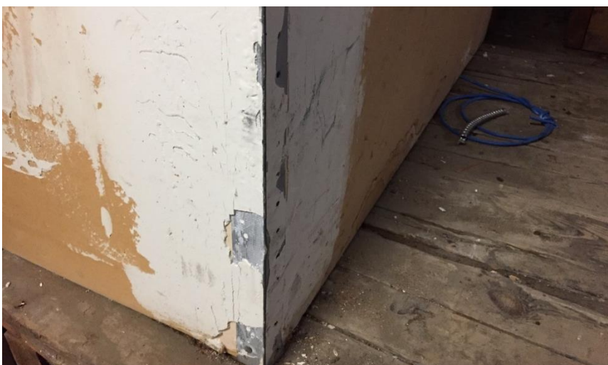
Photo 12: View of the poor condition drywall with asbestos-containing joint compound observed in Room 002.
