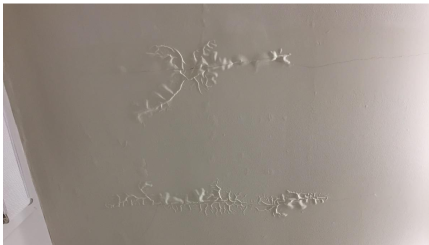
Photo 13: View of the poor condition lead-containing ceiling paint (White) observed in Room 207.
