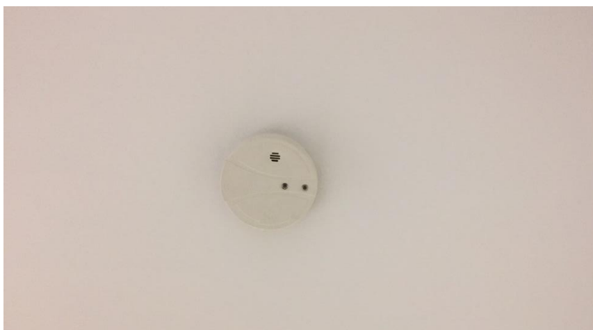
Photo 6: View of the smoke detectors containing radioactive materials observed in Room 001.
