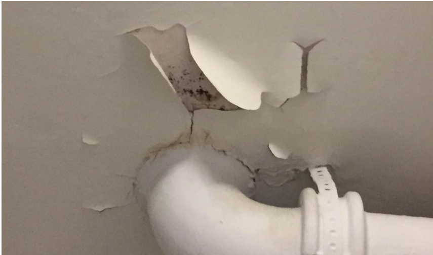
Photo 10: View of the poor condition lead-containing ceiling paint (White) observed in Room 207.
