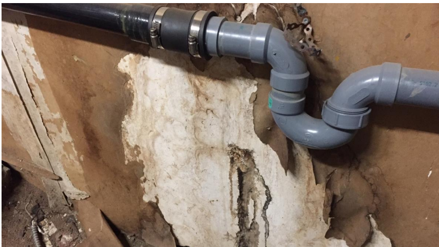
Photo 11: View of the poor condition drywall with asbestos-containing joint compound observed in Room 002A.
