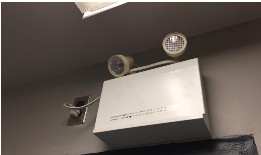
Photo 5: View of the lead-containing battery pack observed in Room 300.
