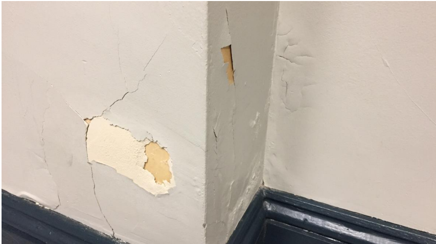
Photo 7: View of the poor condition asbestos-containing drywall joint compound was observed in Room 100D.
