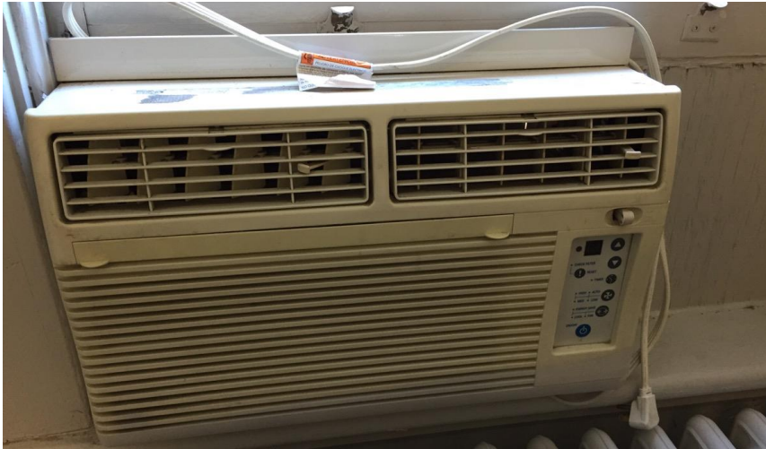
Photo 4: View of the ODS-containing equipment observed throughout the subject building.
