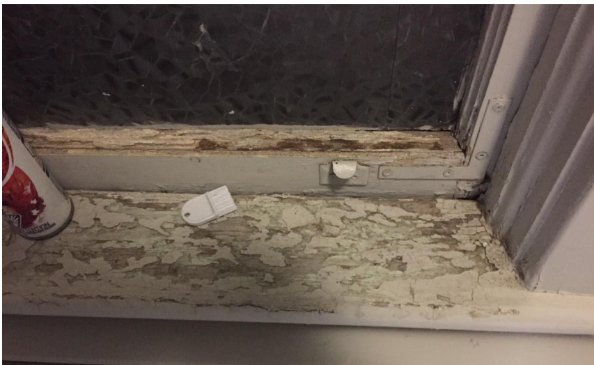
Photo 9: View of the poor condition lead-containing windowsill paint (Grey) observed in Room 303.
