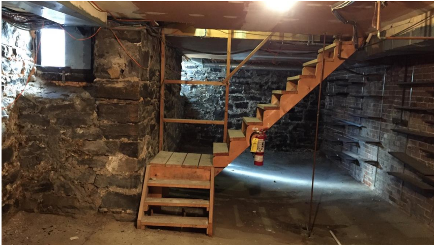
Photo 1: Representative view of the interior finishes observed throughout the subject building basement.
