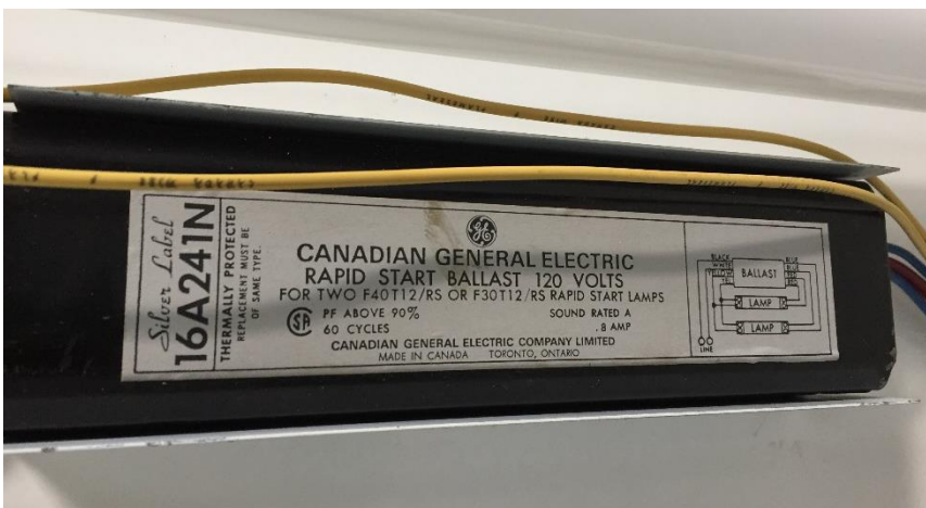
Photo 6: Representative view of the suspected PCB-containing light ballasts observed in the subject building.
