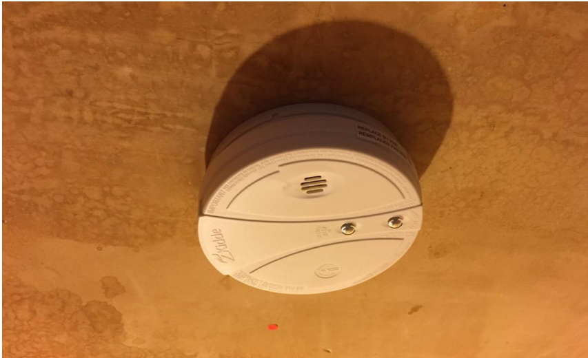
Photo 4: View of the Kidde brand smoke detector containing radioactive materials observed in Room 105A.
