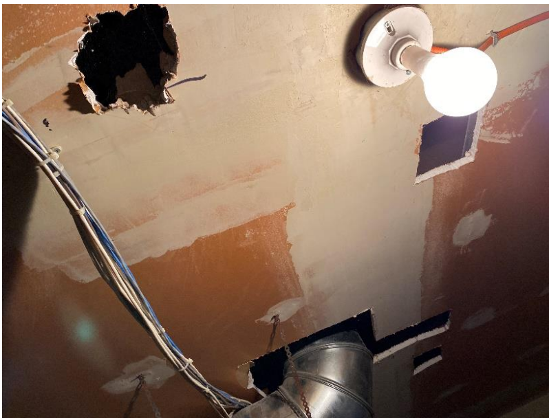
Photo 8: View of asbestos-containing drywall joint compound (ceiling) observed to be in poor condition in Room B1
