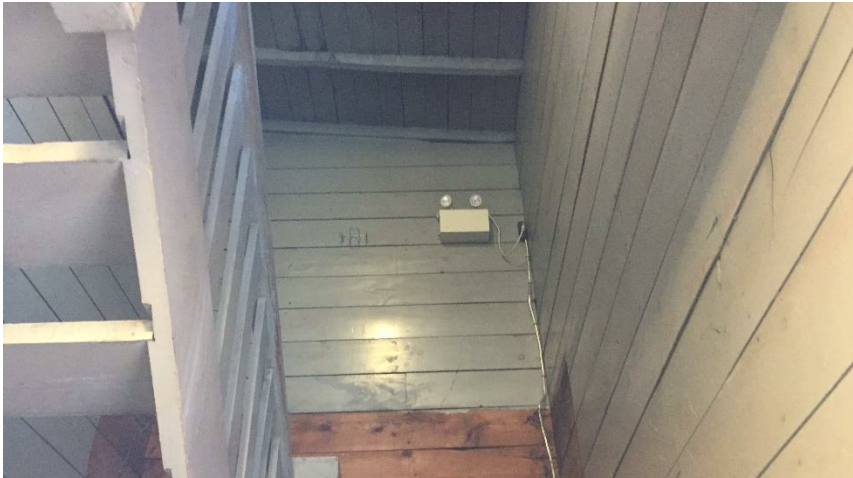
Photo 4: View of lead-containing battery pack observed in emergency lights..
