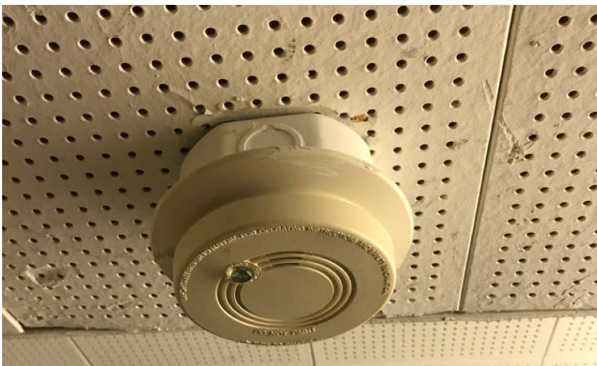
Photo 6: Typical view of radioactive-containing smoke detectors observed throughout the subject building.
