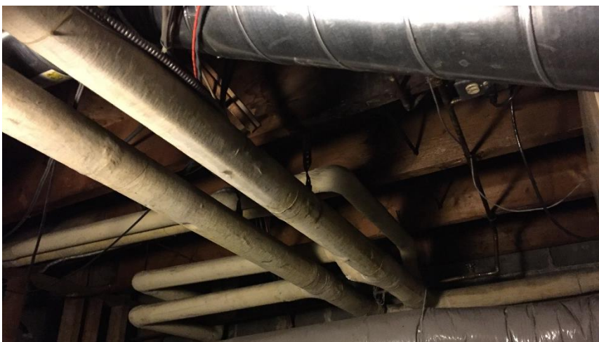
Photo 3: Representative view of the asbestos-containing parging cement elbows and pipe straight insulation observed in Room B10.
