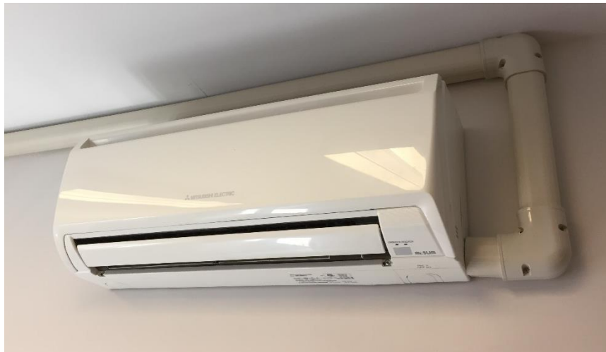
Photo 10: View of the equipment containing ODSs observed throughout the subject building.
