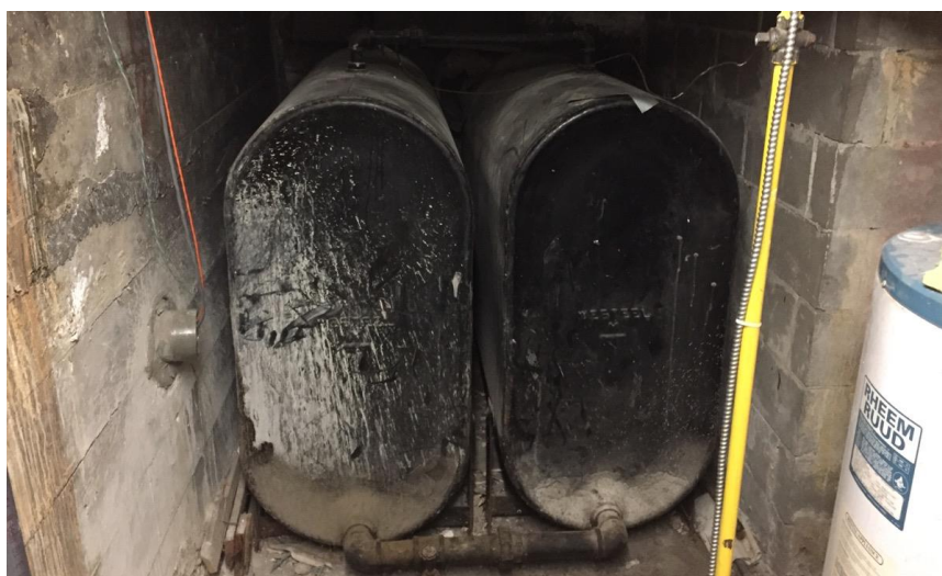
Photo 11: View of the above ground diesel storage tanks identified in Room B8.
