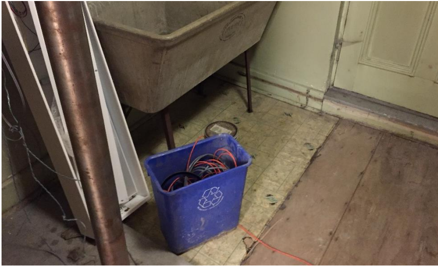
Photo 7: View of the asbestos-containing vinyl sheet flooring (Yellow Rectangular Pattern) observed in Room B9.
