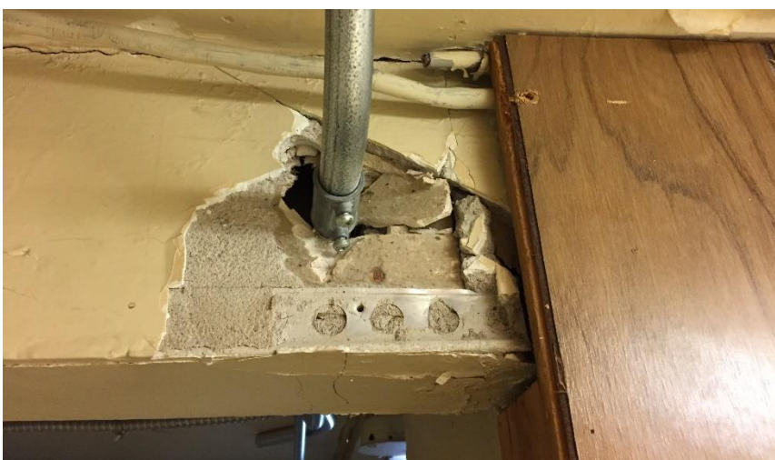
Photo 3: View of the non-asbestos containing wall plaster observed throughout the subject building.
