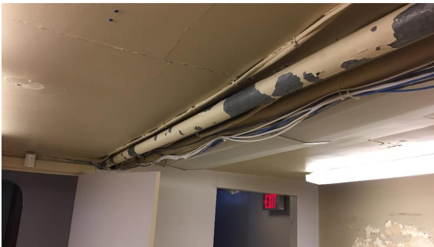
Photo 2: View of the poor condition lead paint (Beige) identified on pipe straights in Room B5.
