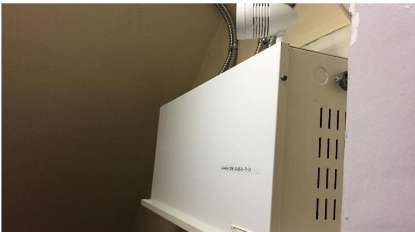
Photo 8: View of the lead-containing batteries observed in Room B2.
