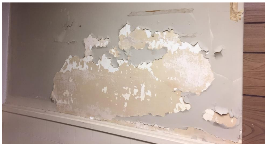
Photo 6: View of the poor condition lead-containing wall paint (Beige) observed in Room B5.
