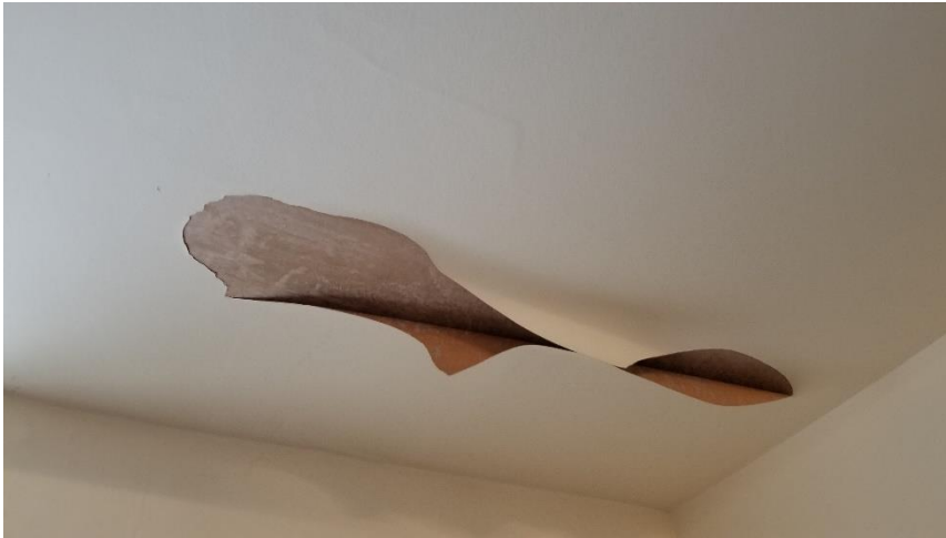
Photo 24: View of the lead-containing ceiling paint (White) observed in poor condition in Room 307.
