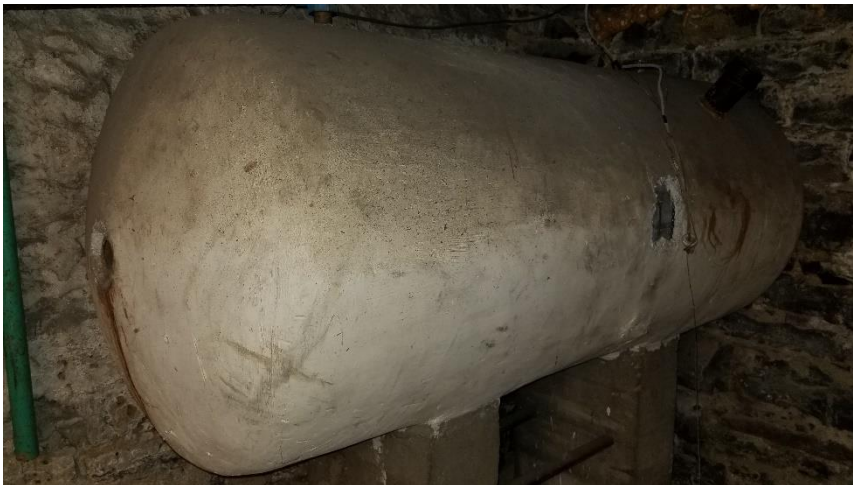
Photo 2: View of the asbestos-containing boiler tank insulation (paring cement) observed in poor condition in Room B5.
