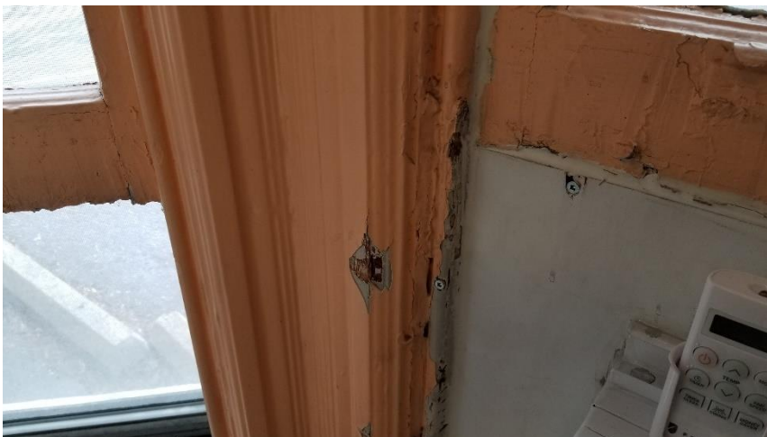
Photo 17: View of the lead-containing frame paint (Peach) observed in poor condition in Room 108.
