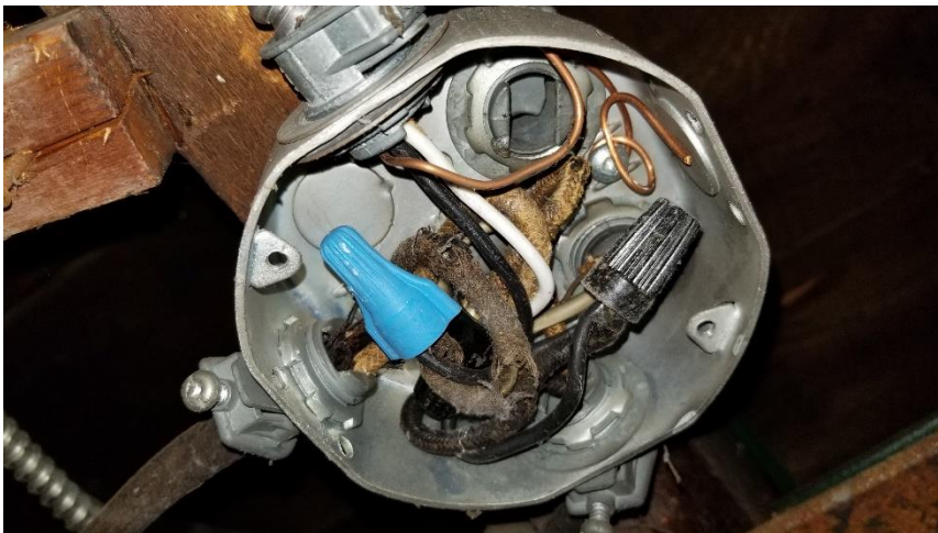
Photo 6: View of the electrical wire fabric cover (Brown) suspected of containing asbestos and PCBs in Room B5.
