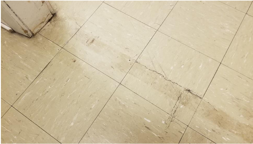
Photo 10: Representative view of the asbestos-containing vinyl floor tiles (12"x12" – Green) observed in fair condition in Room 101.
