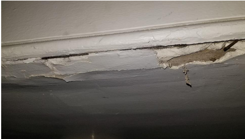
Photo 18: View of the asbestos-containing plaster observed in poor condition in Room 100.
