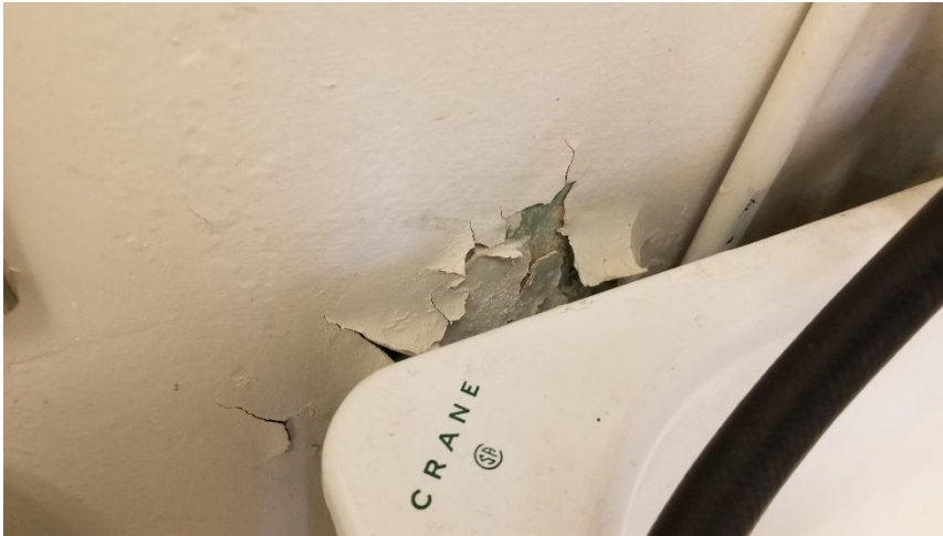
Photo 13: View of the lead-containing wall paint (White) observed in poor condition in Room 103 during the 2022 Reassessment.
