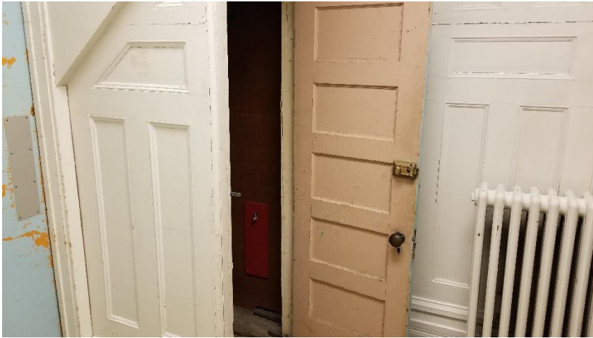
Photo 1: Representative view of the lead-containing light pink door paint identified throughout the first level of subject building in fair condition.
