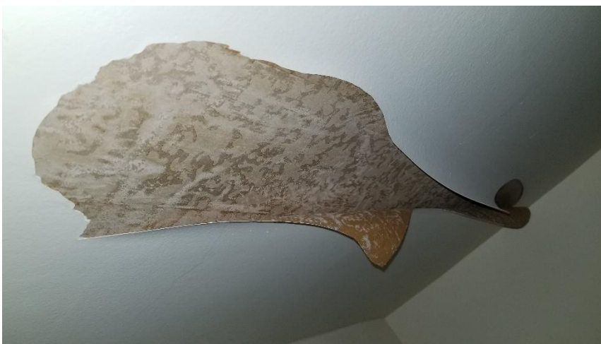
Photo 23: View of the lead-containing ceiling paint (White) observed in poor condition in Room 307C.
