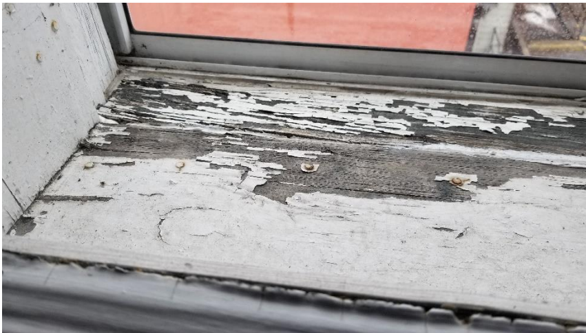
Photo 22: View of the lead-containing window frame paint (White) observed in poor condition in Room 307.
