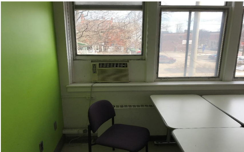
Photo 6: View of air conditioning containing ozone depleted substance in Room 201
