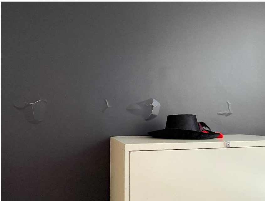
Photo 16: View of asbestos-containing plaster wall observed to be in poor condition in Room 307A during the 2022 Reassessment.
