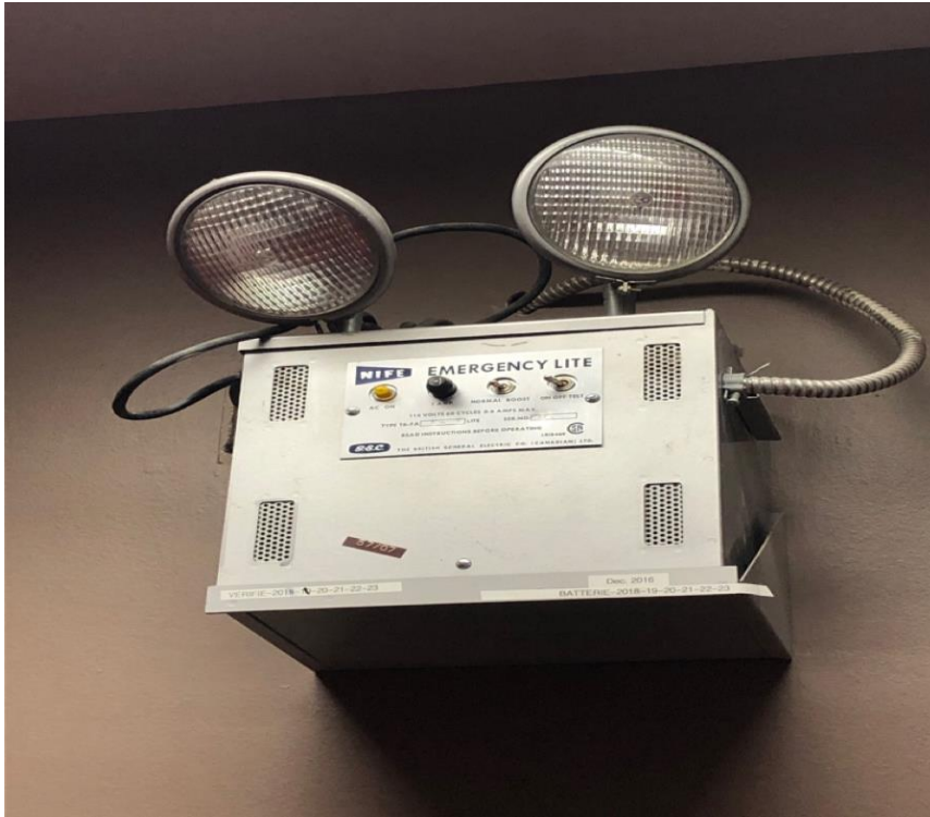
Photo 7: View of lead containing Emergency light in Room 207
