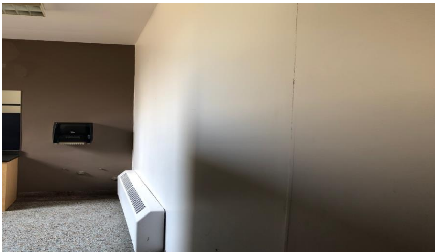
Photo 3: View of asbestos-containing drywall joint compound observed to be in fair condition in Room 202
