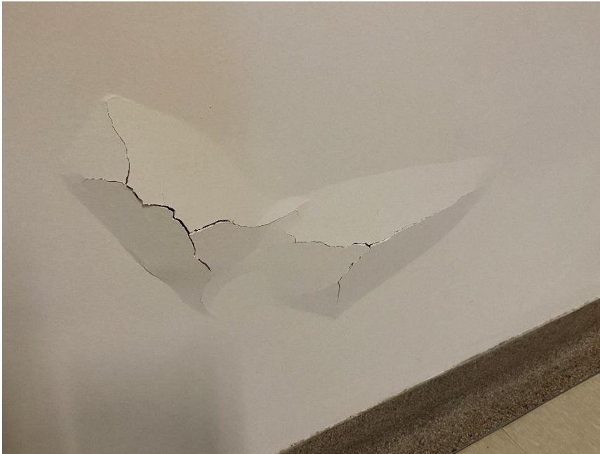
Photo 15: View of asbestos-containing plaster wall observed to be in poor condition in the Hallway adjacent to Room 304 during the 2022 Reassessment.
