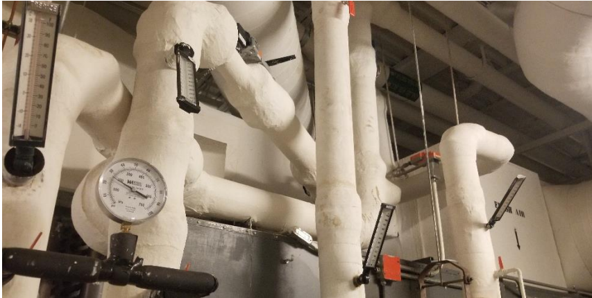
Photo 4: View of mercury-containing pressure gauges and thermometers observed in Room 400.
