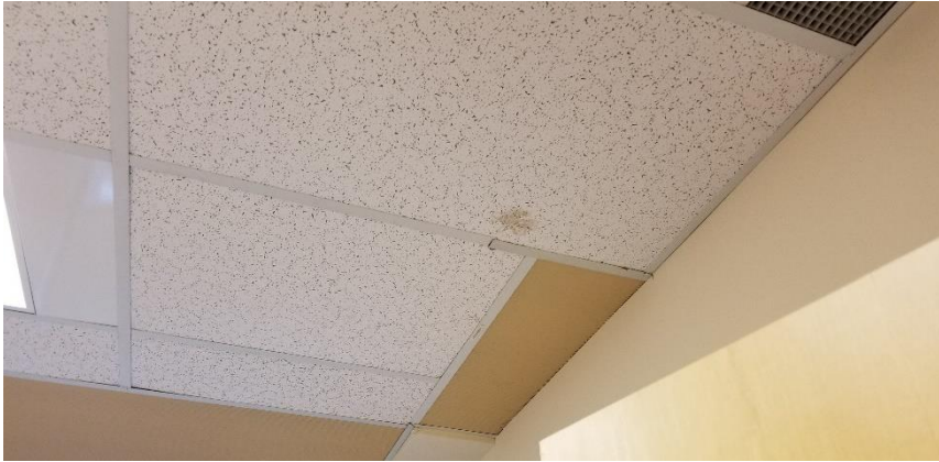
Photo 7: View of water damaged ceiling tiles observed in Room 301E.
