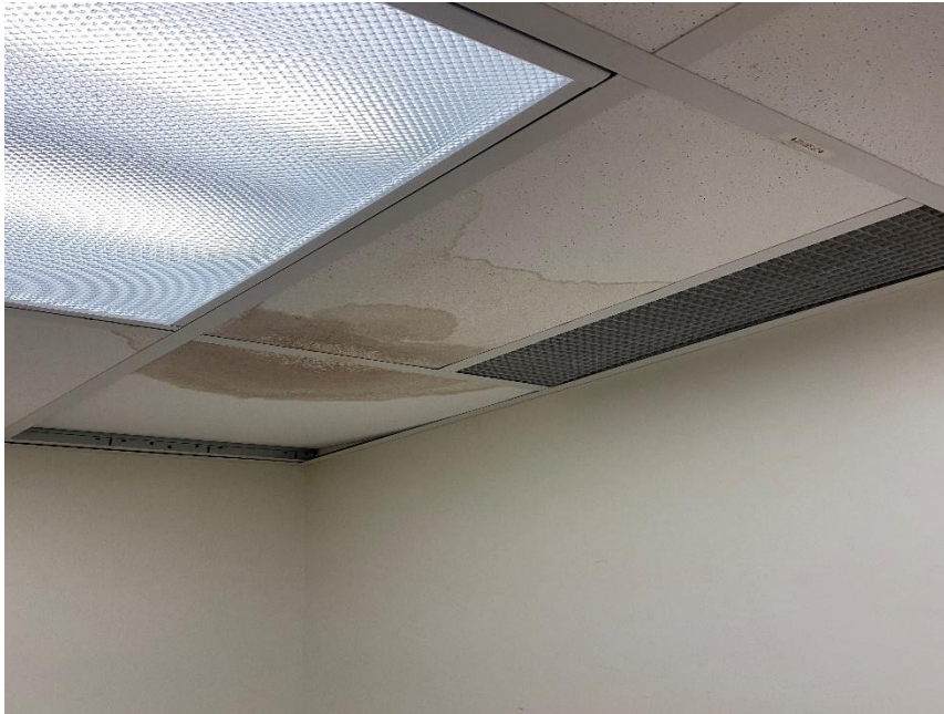
Photo 5: View of water damage observed on suspended ceiling tile.
