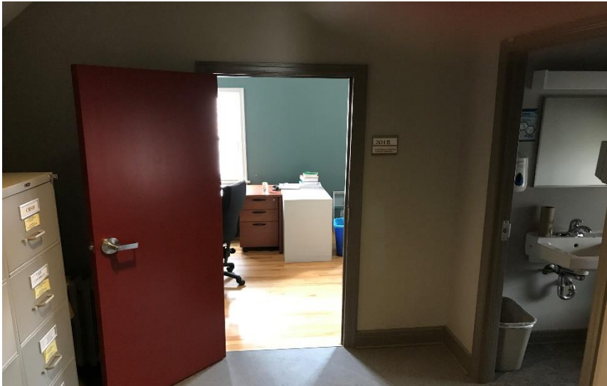
Photo 6: View of red door in Room 201B with low lead concentration.
