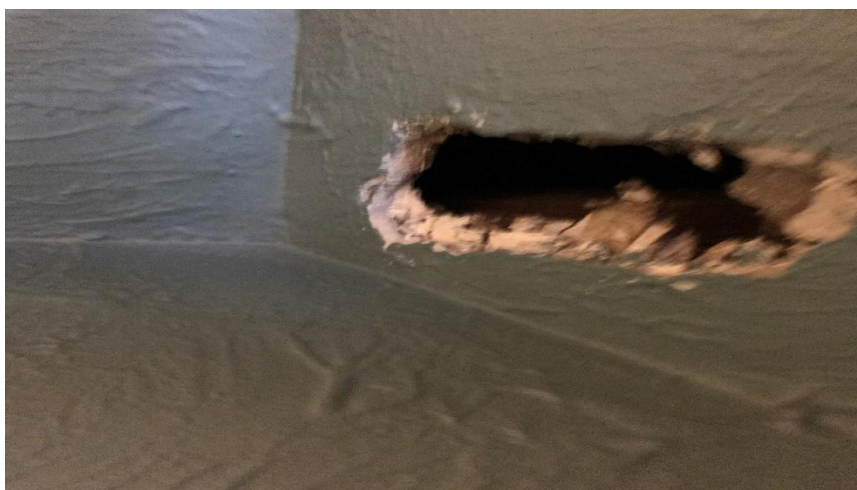
Photo 5: View of asbestos-containing plaster observed to be in poor condition in Room 204A.
