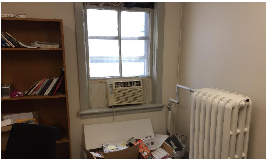
Photo 8: View of the equipment containing ozone depleting substances, observed throughout the subject building.
