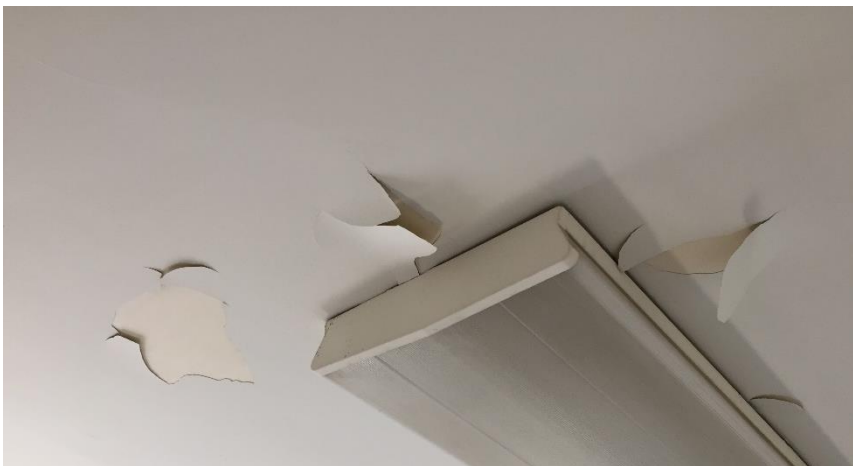
Photo 7: View of the poor condition lead paint (White) observed in Room 307
