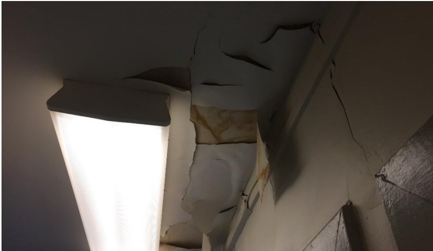
Photo 6: View of the poor condition lead paint (White) and water damaged drywall observed in Room 301
