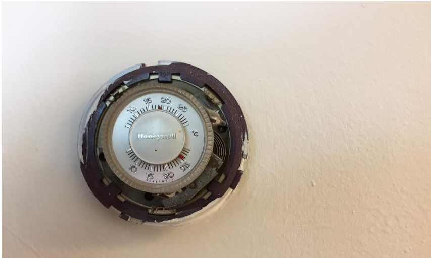
Photo 4: View of the Honeywell thermostat containing liquid mercury, observed in Room 103.
