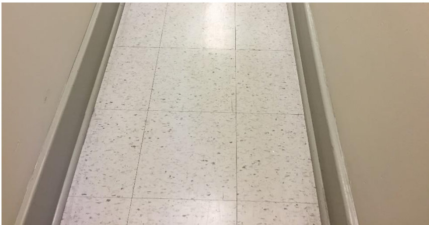
Photo 10: View of the non-asbestos containing vinyl floor tiles (12"x12" White with Light and Dark Grey Flakes) observed throughout the subject building.
