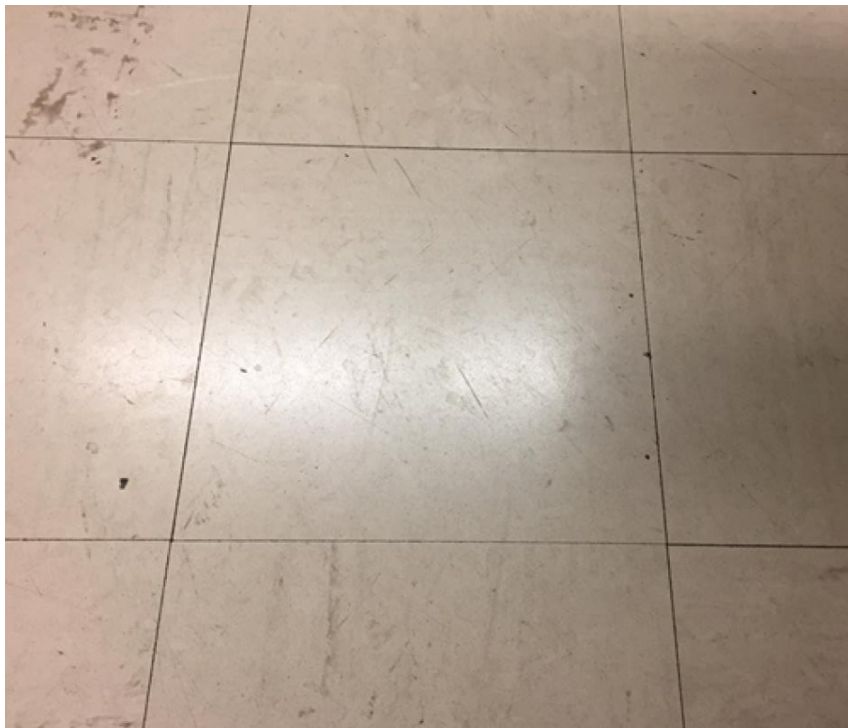
Photo 2: View of asbestos-containing vinyl floor tiles observed in Room M12 of Subject Building.
