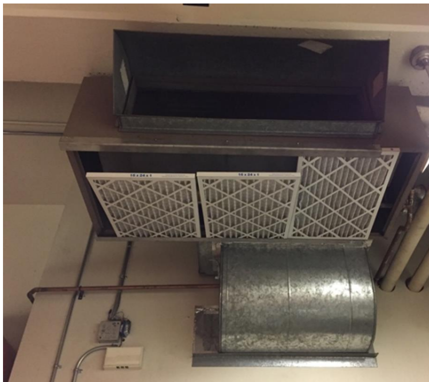
Photo 6: View of ODS Air Conditioning Unit observed in Room M13A of Subject Building.
