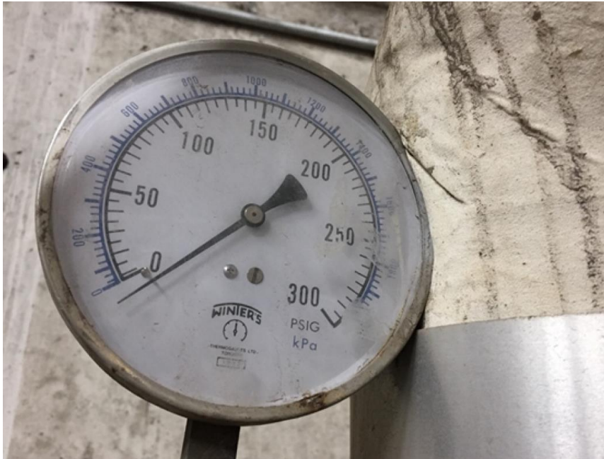
Photo 7: View of Winters' Pressure Gauge observed in Room 008 of Subject Building.
