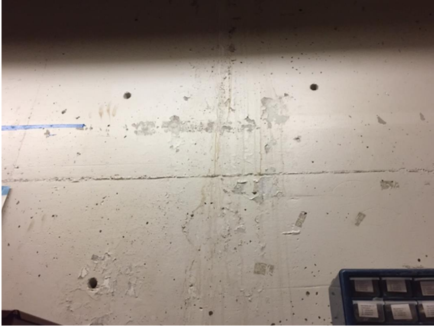
Photo 3: View of poor condition white wall paint observed in Room M13. Sample PB1
