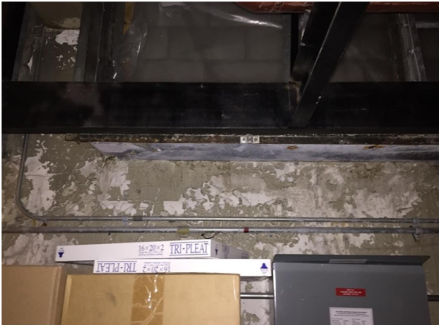
Photo 4: View poor condition grey wall paint observed in Room M09. Sample PB6
