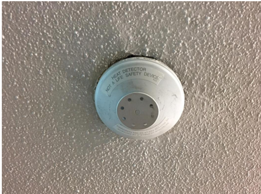
Photo 5: View of Radioactive Smoke Detector observed in Room M03 of Subject Building.
