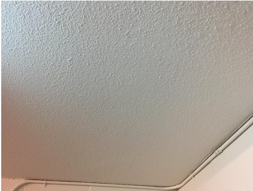
Photo 1: View of asbestos-containing textured ceiling observed in Room M03, M10, M11, and M12 of Subject Building.
