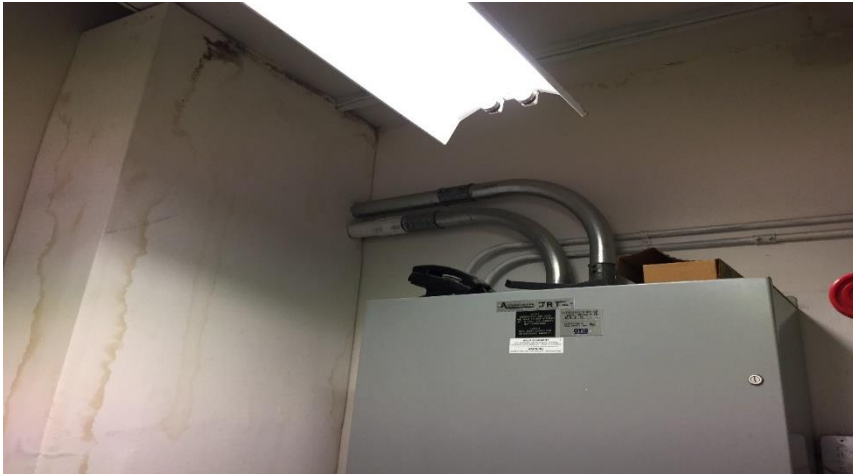
Photo 4: View of suspect mould growth observed on drywall in Room 100D.
