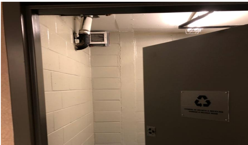
Photo 6: Typical view of light brown door and doorframe paint suspected of containing lead.
