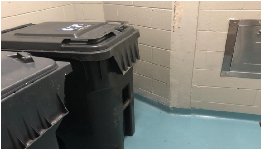
Photo 5: Typical view of teal floor paint and beige wall paint suspected of containing lead.
