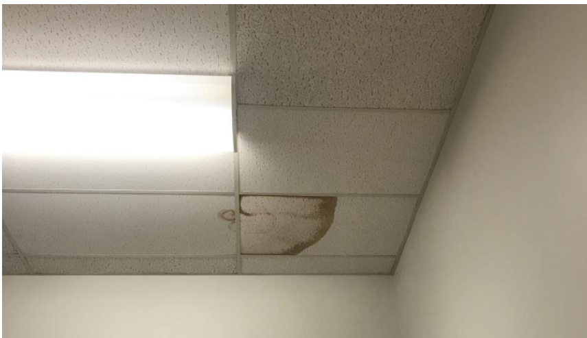
Photo 15: View of water damaged suspended ceiling tile observed in Room 225.
