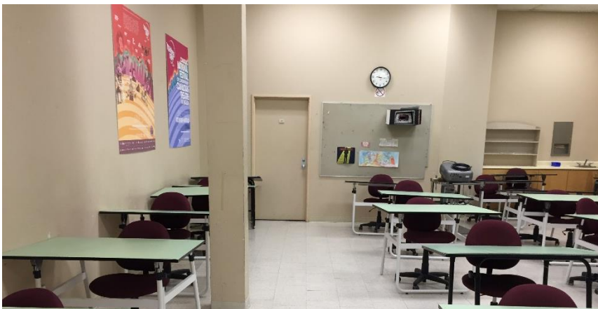
Photo 12: View of asbestos-containing drywall joint compound in Room 202.
