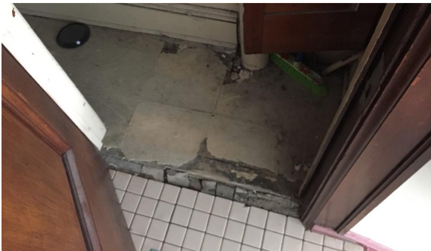
Photo 3: View of asbestos-containing vinyl floor tile observed to be in poor condition within Room 110A.
