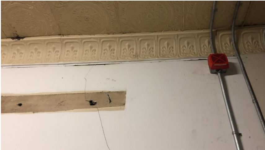
Photo 13: View of damaged asbestos-containing wall/ceiling plaster from Room 400.
