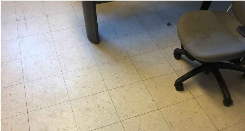
Photo 4: View of Asbestos-containing vinyl floor tiles in Room 107.
