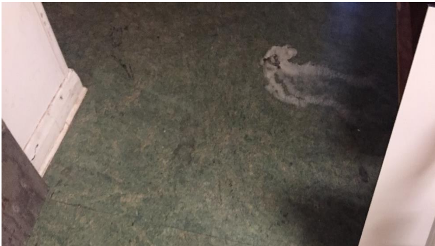
Photo 8: View of vinyl sheet flooring associated with asbestos-containing loose fibres in Room 400.
