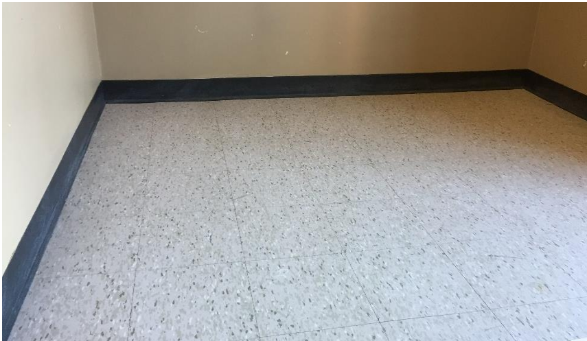
Photo 2: View of asbestos containing vinyl floor tile observed in Room 103.
