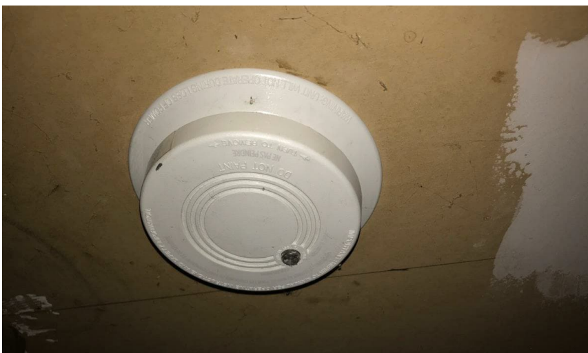
Photo 6: Representative view of the smoke detectors containing radioactive materials observed throughout the subject building.
