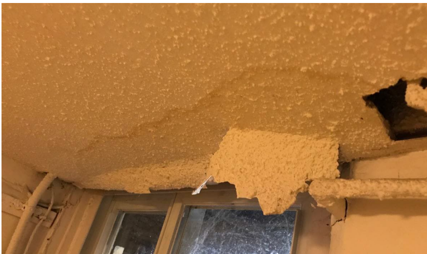
Photo 8: View of the water damaged ceiling observed in Room 06.
