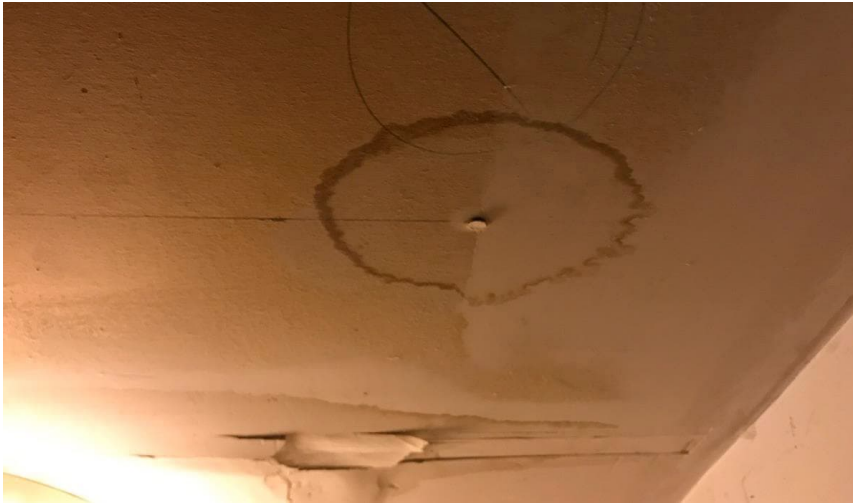
Photo 7: View of the water damaged drywall ceiling observed in Room 03.
