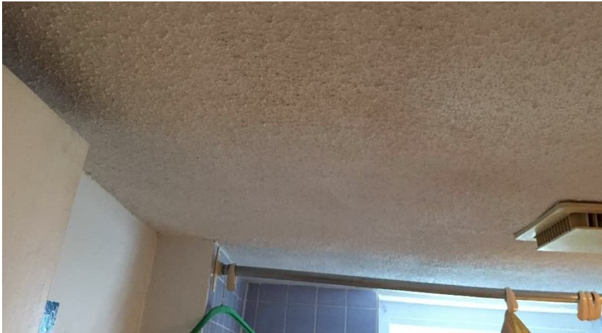
Photo 4: View of the non-asbestos-containing ceiling texture coat observed throughout the subject building.
