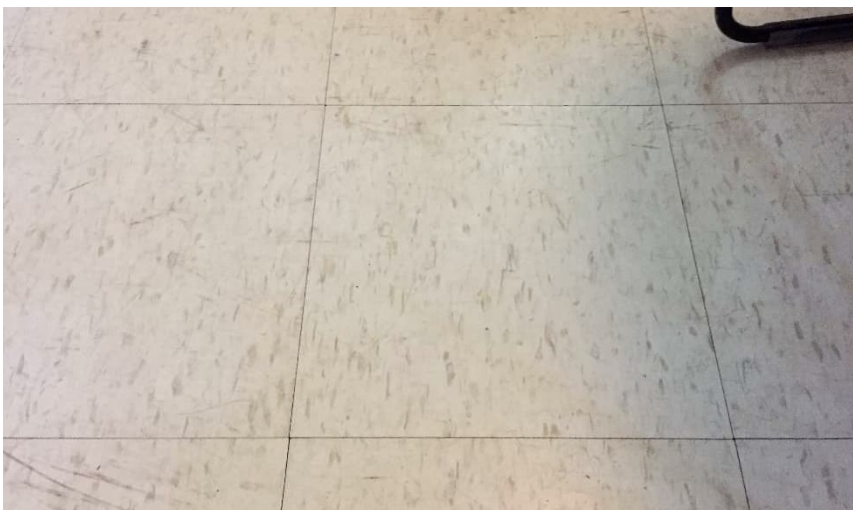
Photo 2: View of the non-asbestos-containing vinyl floor tiles (12"x12" - White with Beige Flakes) observed in Room 12.
