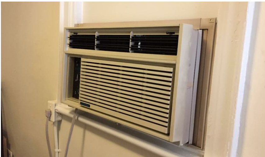
Photo 5: View of the ODS-containing equipment observed throughout the subject building.
