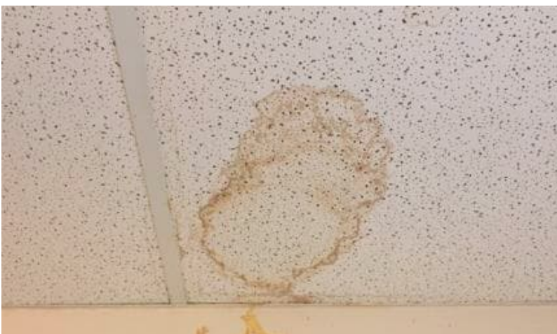
Photo 6: View of water damaged ceiling tile observed in the kitchen.
