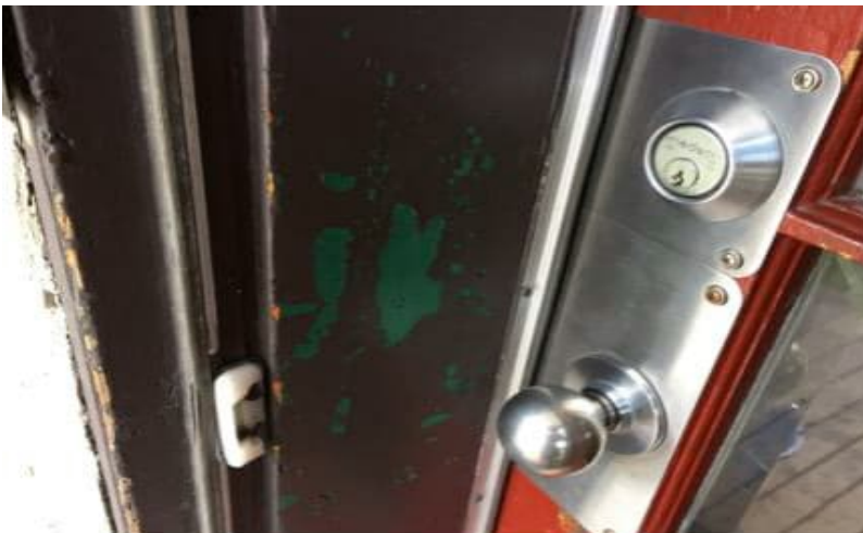
Photo 5: View of lead-containing dark grey paint observed to be in poor condition on the front door.
