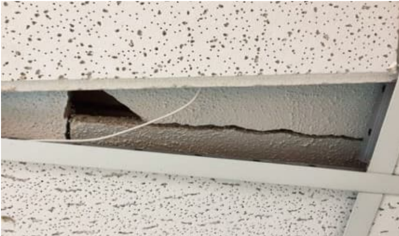
Photo 4: View of suspended ceiling tiles with a ceiling texture coat above, as observed in Room A on the second floor.
