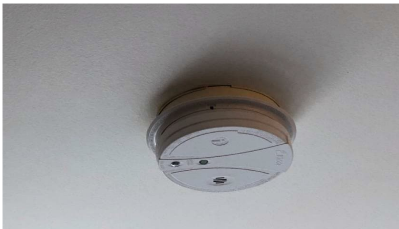
Photo 9: Typical view of smoke detectors containing radioactive materials.
