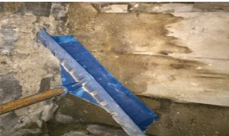
Photo 9: View of water-damaged wood stairs in the basement.
