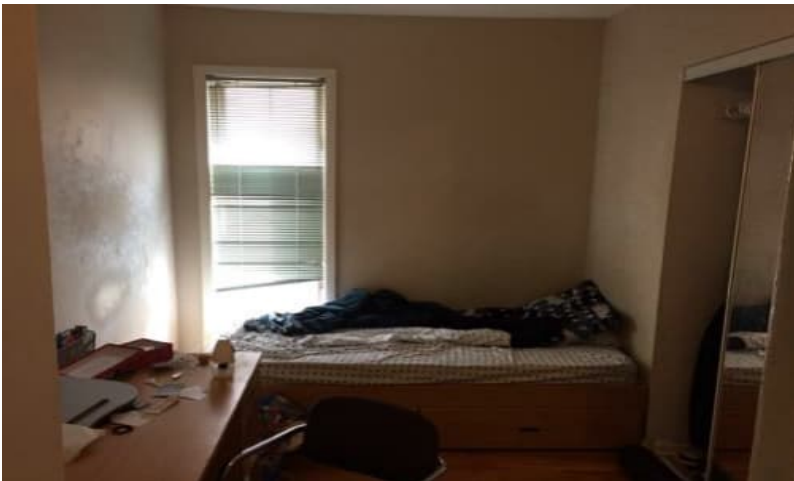
Photo 2: View of typical finishes observed at the building located at 122 Henderson Avenue.
