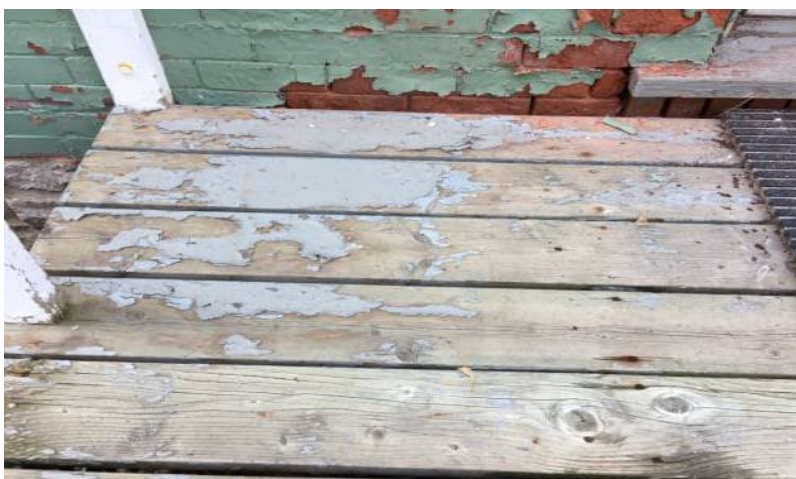
Photo 6: View of lead-containing grey and green paint observed to be in poor condition on the front deck.
