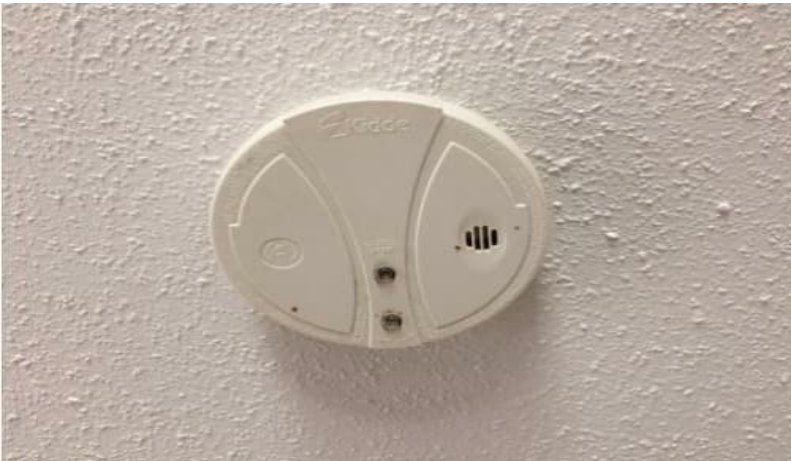
Photo 8: Typical view of smoke detectors containing radioactive materials.
