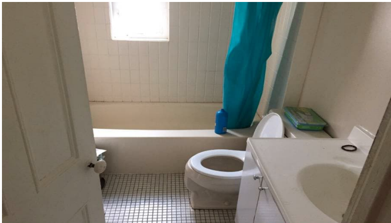
Photo 5: Typical view of ceramic wall/floor tile grout suspected of containing asbestos.
