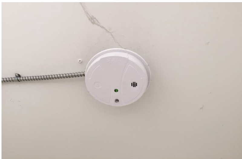
Photo 10: Typical view of smoke detectors containing radioactive materials.
