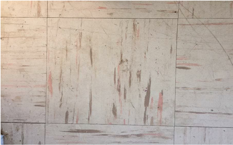
Photo 4: View of asbestos-containing vinyl floor tiles (9"x9"- Beige with Pink and Brown Streaks) observed in Room B on the 2 nd Floor.
