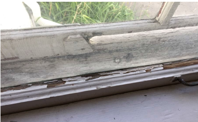
Photo 9: View of lead-containing white paint observed to be in poor condition in the kitchen on the 1 st floor.
