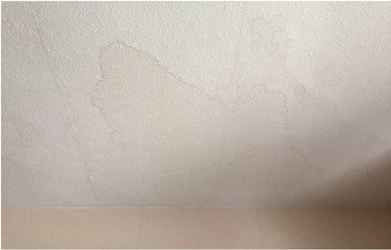
Photo 7: View of water-damaged texture coat observed in Room B on the 1 st Floor.
