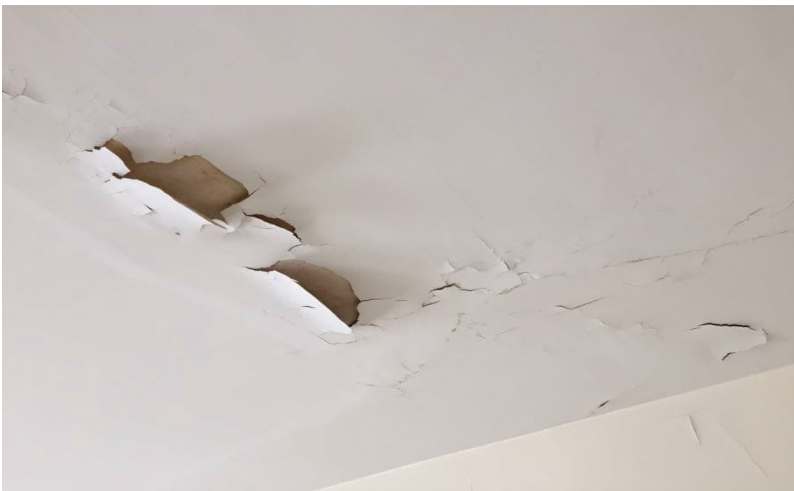
Photo 8: View of lead-containing white paint observed to be in poor condition in Room D on the 2 nd floor.
