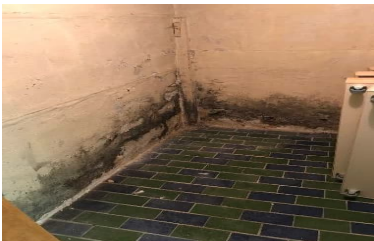
Photo 3: View of suspect mould growth observed on concrete walls in the basement of the subject building.
