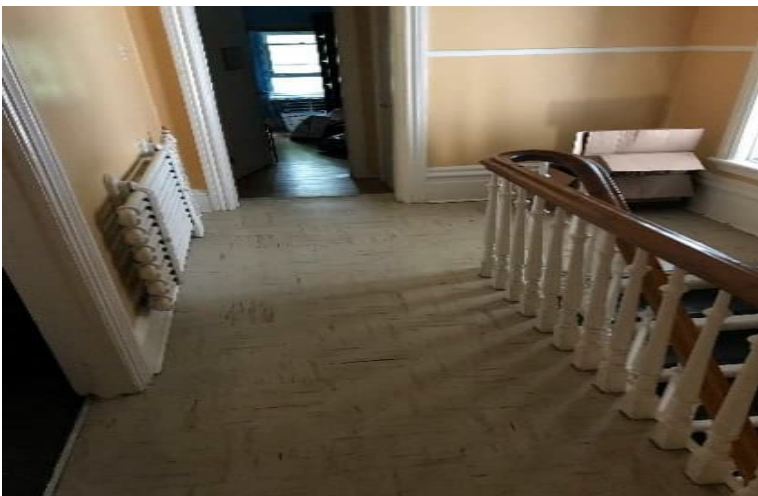
Photo 2: View of asbestos-containing vinyl floor tile observed in the 1 st floor landing.
