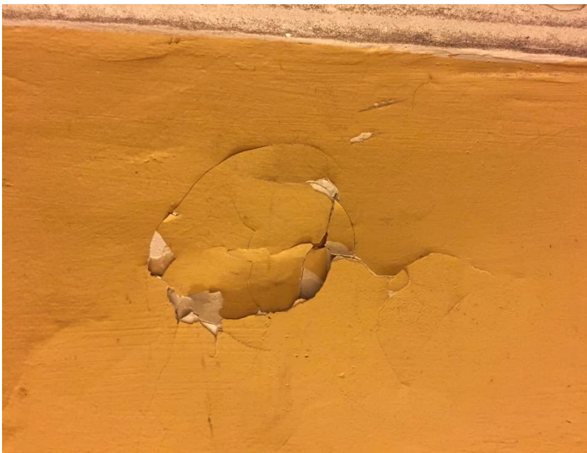
Photo 6: View of the poor condition asbestos-containing plaster and lead paint observed in Room 100A of 15 Stewart Street.
