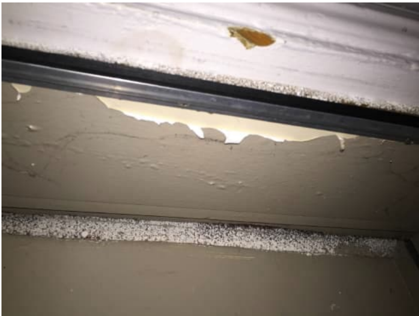
Photo 8: View of the poor condition lead-containing door frame paint observed in Room 108/112 of 17 Stewart Street.
