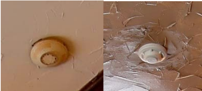
Photo 7: View of smoke detectors with radioactive material present throughout the building.
