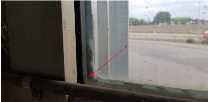
Photo 1: View of asbestos-containing interior window caulking (black) observed to be in good condition in Room 139.
