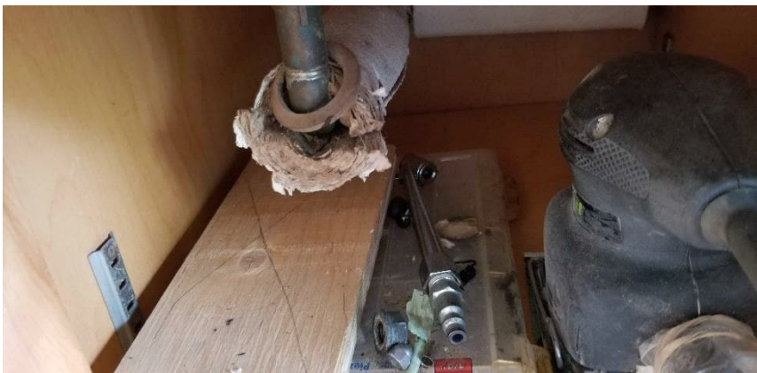
Photo 3: View of asbestos-containing mechanical pipe straight insulation observed to be in poor condition on the 2 nd work bench outside the bike shop office in Room A 105.
