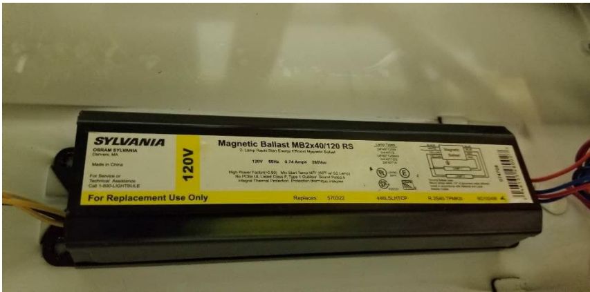
Photo 17: Typical view of non-PCB containing light ballast observed throughout the surveyed building.
