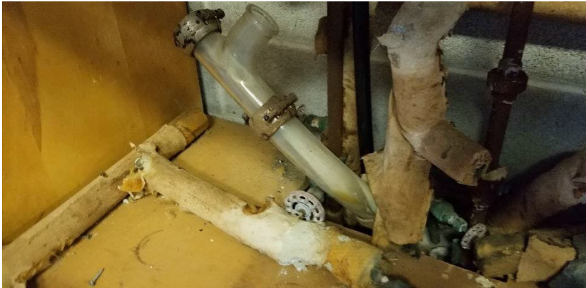
Photo 4: View of asbestos-containing mechanical pipe fittings observed to be in poor condition in Room A104. This damage has been repaired.
