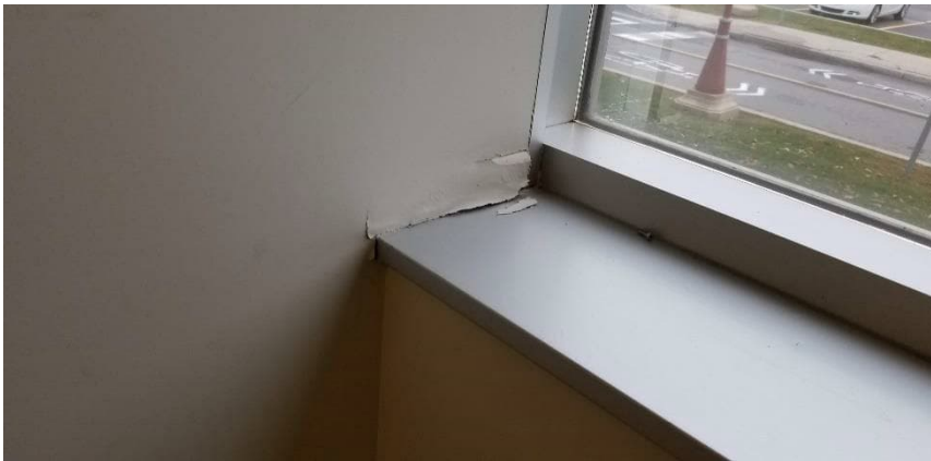
Photo 14: View of water damage on drywall observed in Room E117.
