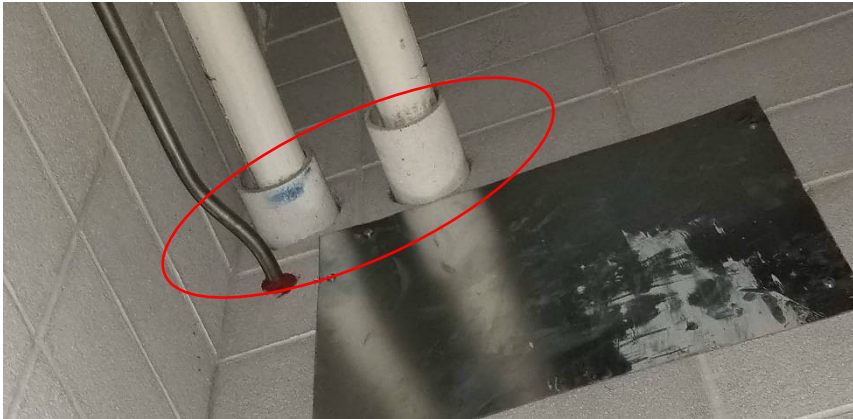
Photo 7: View of asbestos-containing transite pipe (highlighted in red) observed to be in good condition Mechanical Room A138C.
