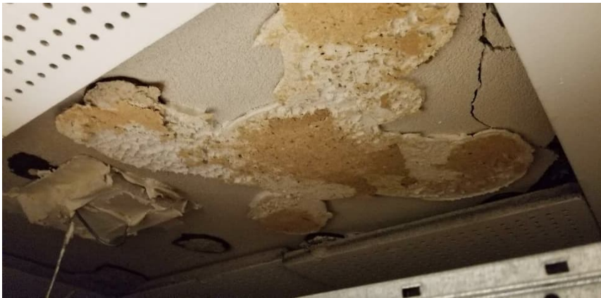
Photo 11: View of non-asbestos-containing glued-on acoustic tile (12"x12"-Uniform Holes) and adhesive mastic (brown) observed in the Men's Change Room in D108.
