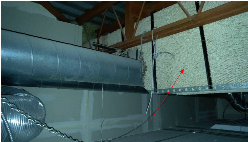
Photo 5: View of asbestos-containing plaster on steel mesh observed in Room B 215N.
