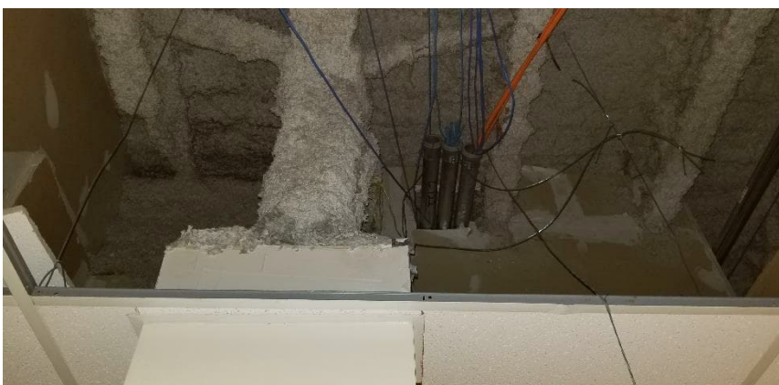
Photo 9: View of non-asbestos-containing fireproofing observed above the suspended ceiling tiles in Room C141C.
