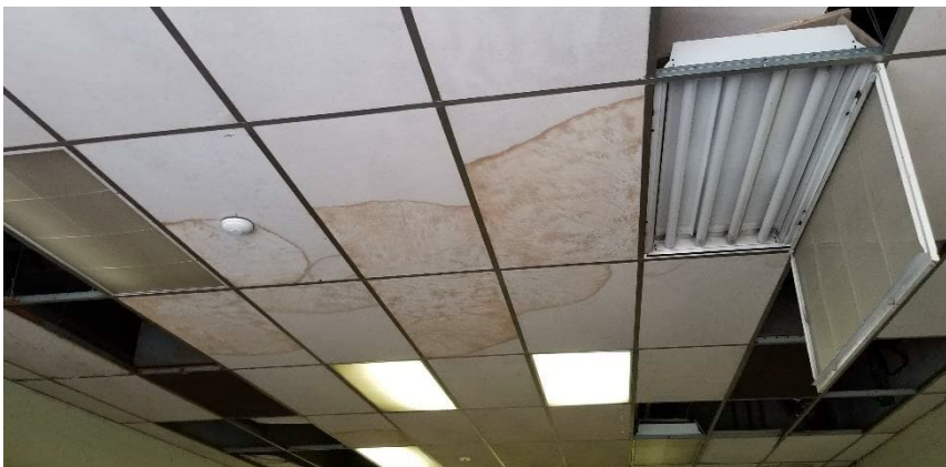
Photo 18: View of water-stained suspended ceiling tiles in Room A104C.
