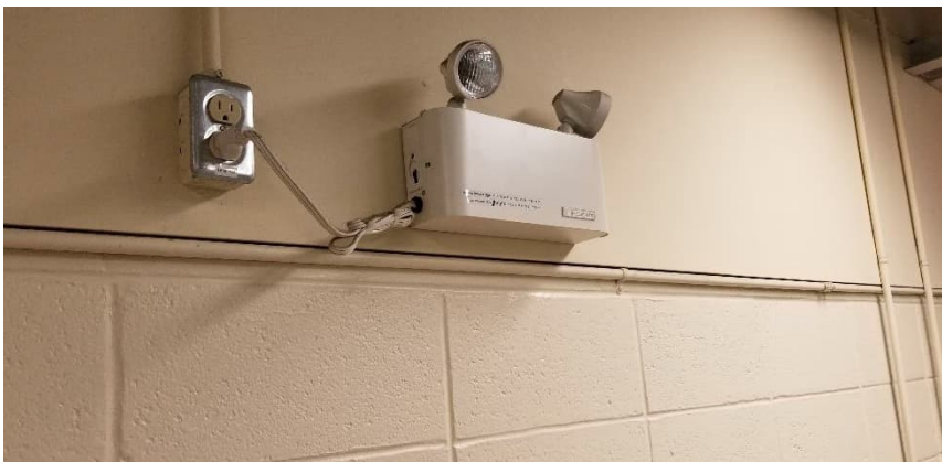
Photo 15: View of lead acid battery pack observed outside of D201.
