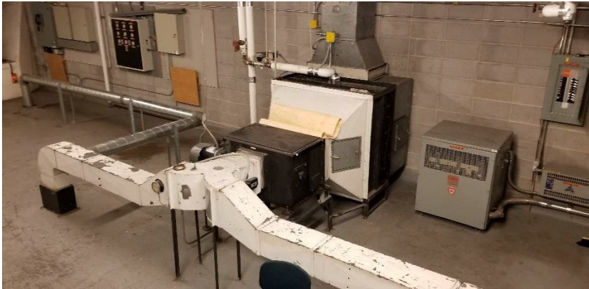
Photo 13: View lead containing white paint was observed to be in poor condition in Mechanical Room D201.
