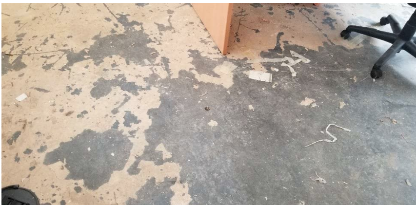
Photo 12: View of low-level lead paint observed to be in poor condition in Room A144.
