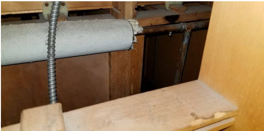
Photo 2: View of asbestos-containing mechanical pipe straight insulation observed to be in poor condition in cabinet 510 in Room A 105.
