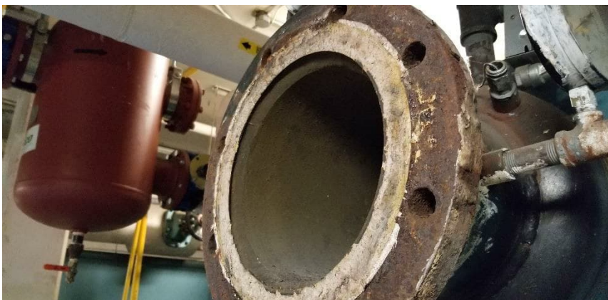
Photo 6: View of asbestos-containing pipe gasket observed on the Unilux Boiler in Mechanical Room A02.
