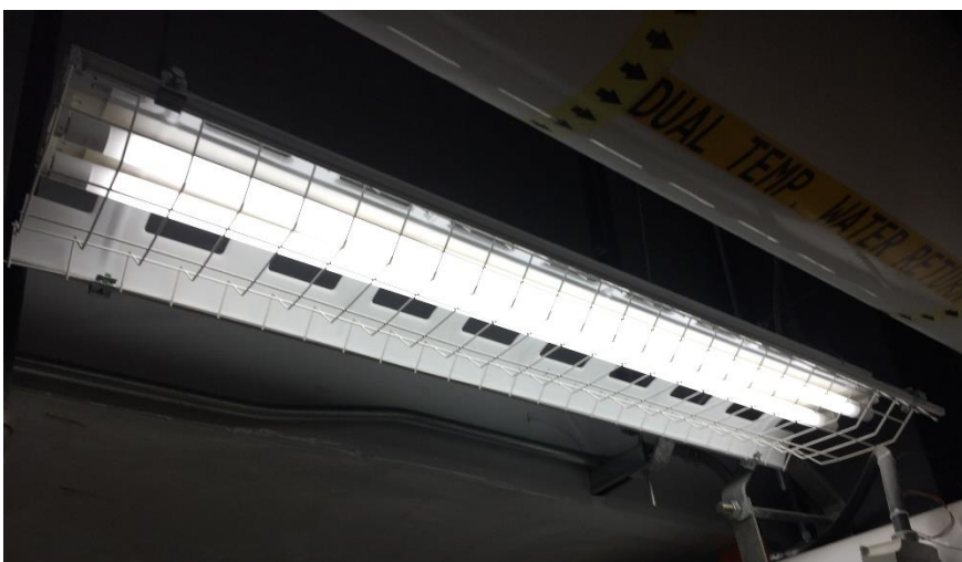
Photo 9: Representative view of the fluorescent light fixtures containing mercury vapour observed throughout the subject building.
