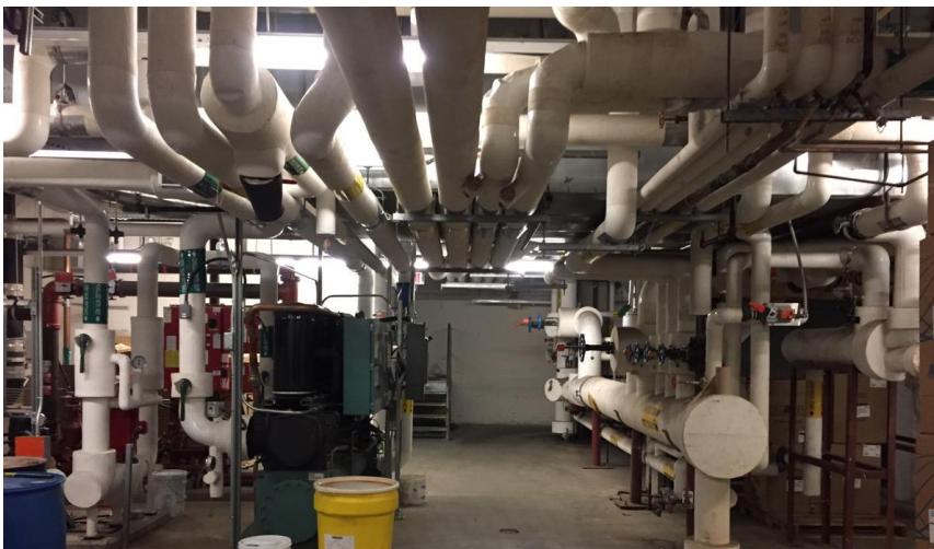
Photo 3: Representative view of the non-asbestos-containing mechanical insulation observed throughout the subject building.
