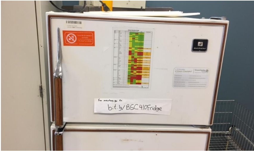
Photo 7: A representative view of the equipment containing ODSs was observed throughout the subject building.
