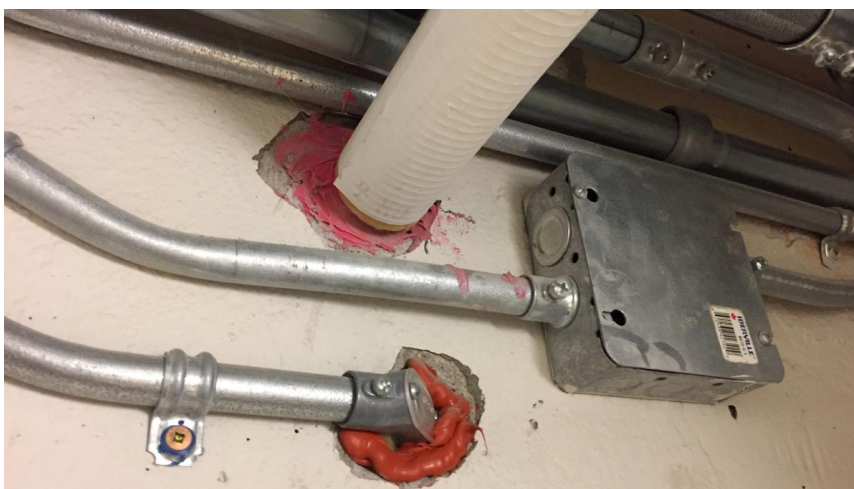
Photo 6: View of the non-asbestos-containing firestop caulking (Red) observed throughout the subject building.
