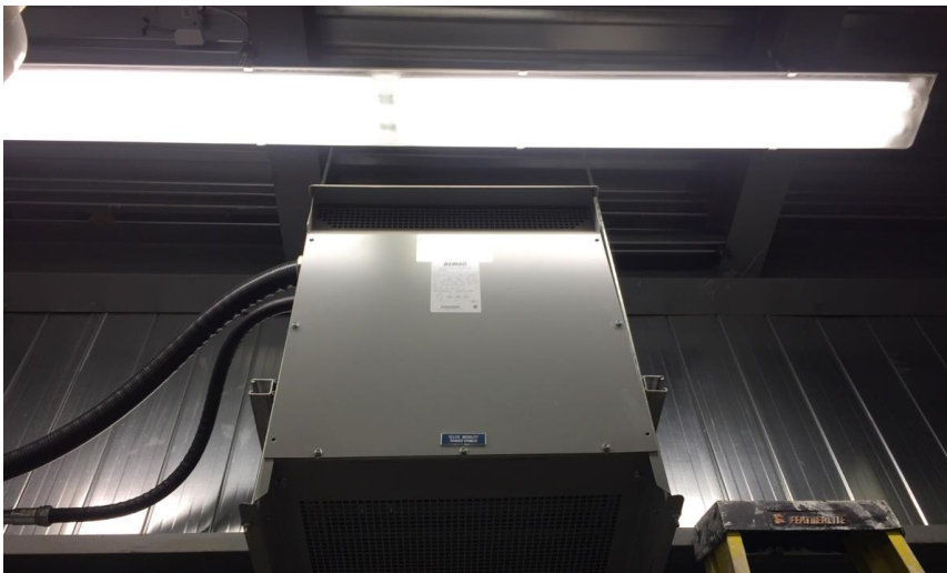
Photo 8: Representative view of the non-PCB dry-type transformers observed throughout the subject building.
