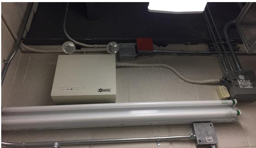
Photo 5: View of the lead-containing battery packs and mercury-containing fluorescent light fixtures observed throughout Room 528.
