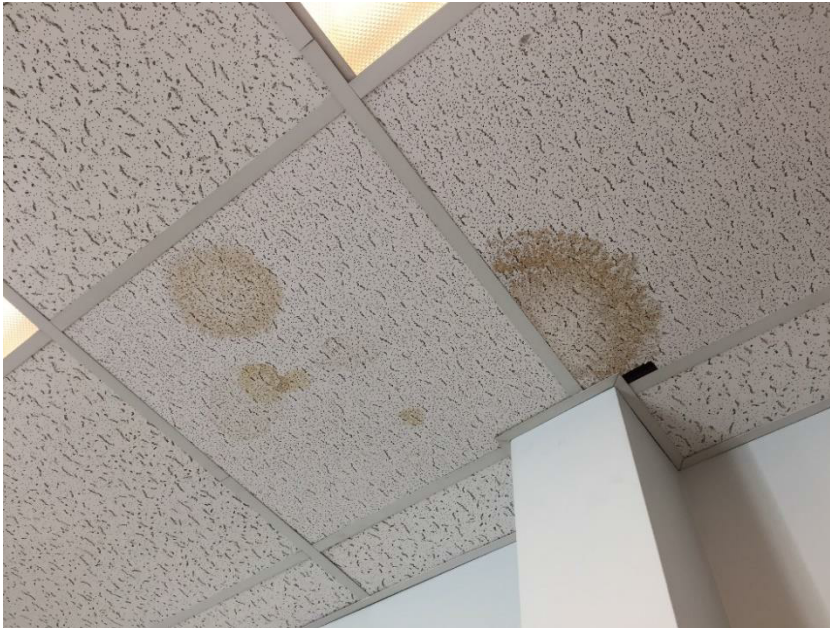
Photo 9: View of water damaged suspended ceiling tiles observed in Room 206.
