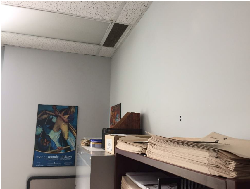
Photo 6: View of asbestos-containing drywall within Room 101
