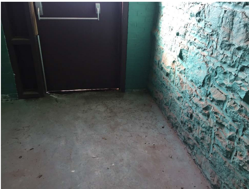
Photo 8: View of lead-containing green paint within the subject building
