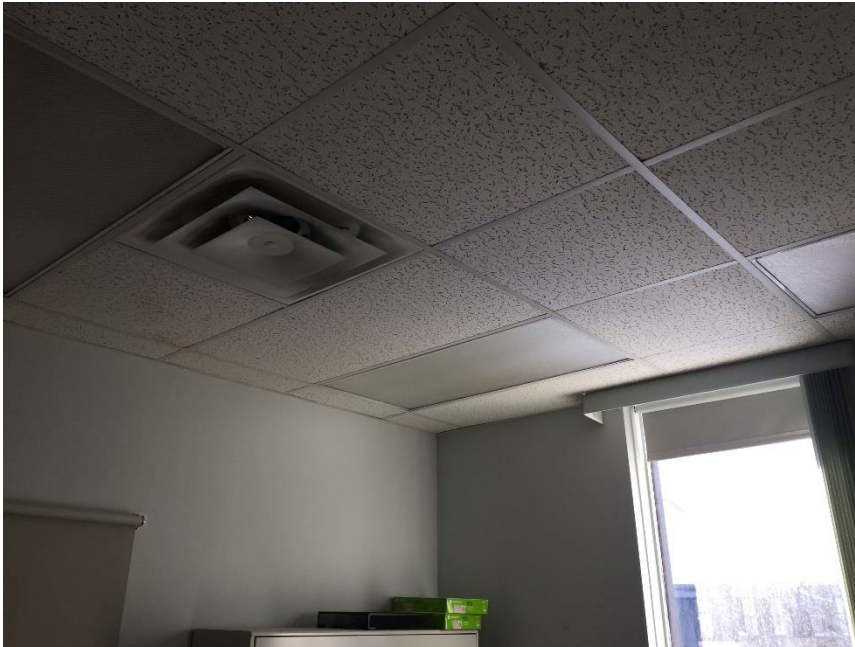
Photo 1: Typical view of non-asbestos-containing suspended ceiling tiles with medium fissure observed within Room 105.
