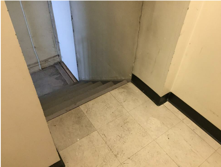
Photo 3: View asbestos-containing vinyl floor tile (beige with brown) within Room 106
