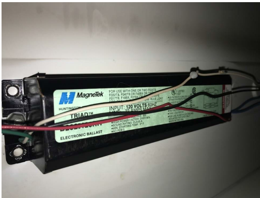
Photo 10: View of non-PCB containing light ballasts observed in Room 0018.
