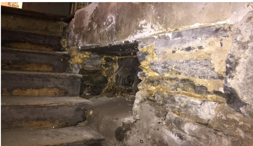
Photo 3: View of lead-containing paint (Grey) on plaster in poor condition in the Basement Room 003.
