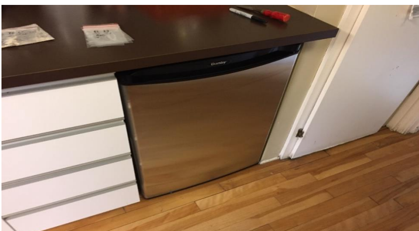
Photo 9: View of equipment observed to contain ODSs in Room 201.
