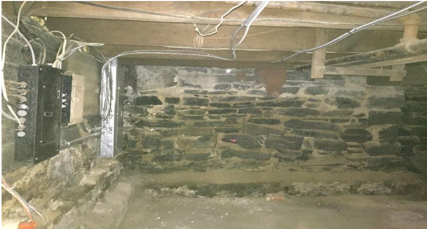
Photo 4: View damp staining on stone foundation wall in the Basement level.
