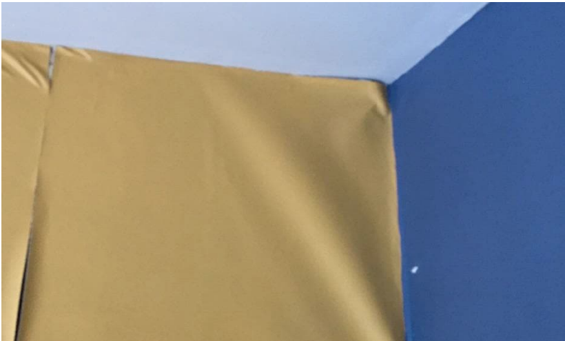
Photo 5: View of lead-containing yellow paint observed to be damaged in Room 203.
