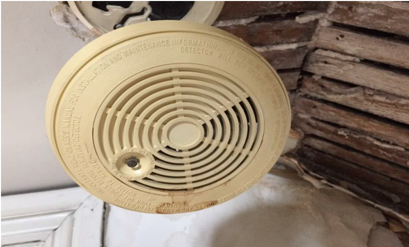
Photo 7: Typical view of radioactive smoke detectors observed within the subject building.
