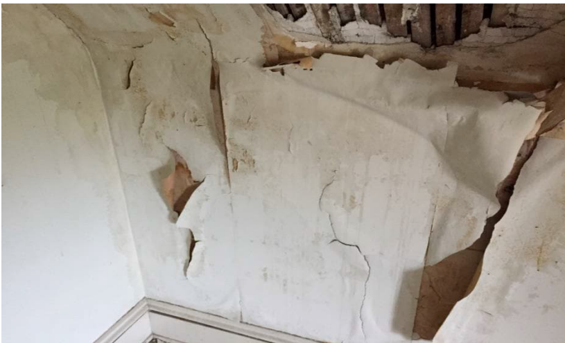
Photo 3: View of white low levels of paint observed to be damaged in Room 302.
