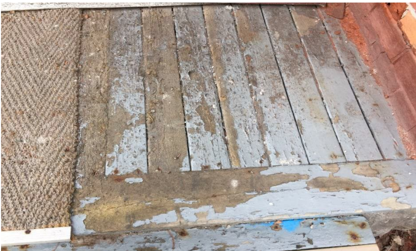
Photo 6: View of lead-containing grey/blue paint observed to be damaged on the exterior deck.
