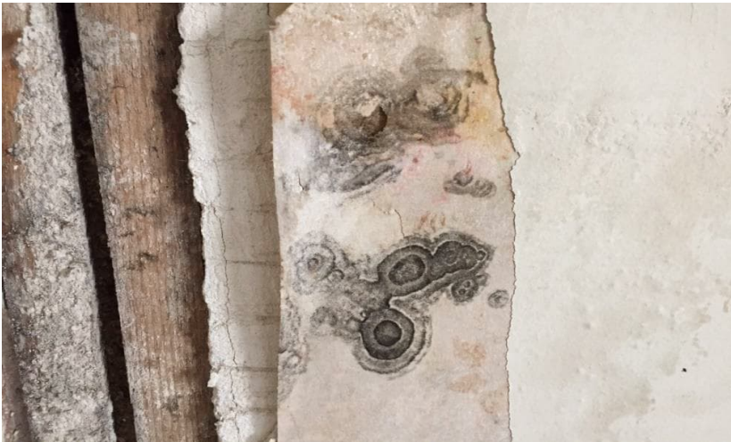
Photo 8: View of suspected mould growth observed on the plaster wall in Room 302.
