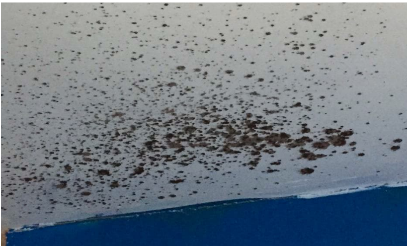
Photo 9: View of suspected mould growth observed on plaster ceiling in Room 202.
