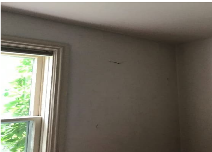
Photo 3: View of lead-containing beige paint observed to be in fair condition in the living room of the subject building.
