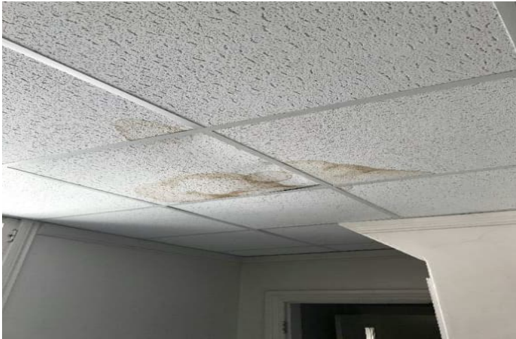
Photo 1: View of water-damaged suspended ceiling tiles (2'x2') observed at 550 King Edward Avenue.
