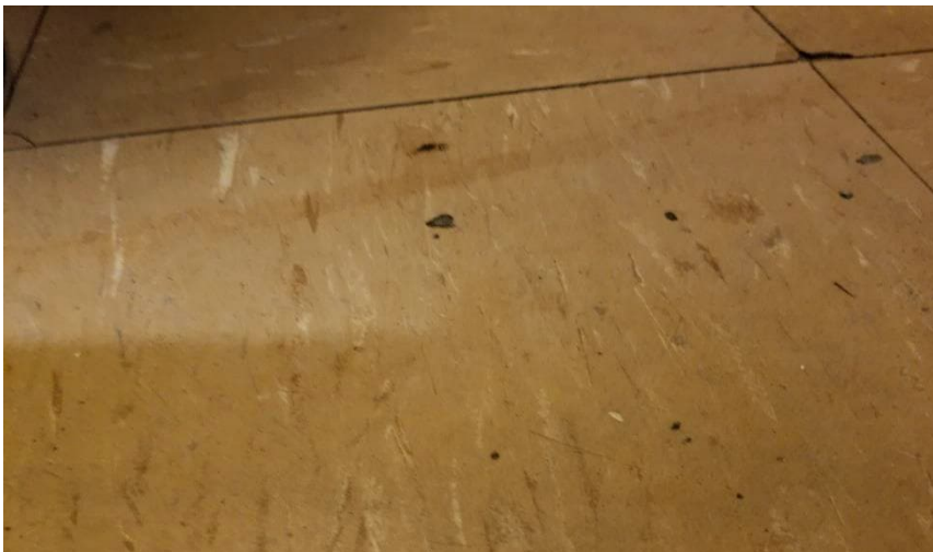
Photo 2: View of asbestos-containing vinyl floor tiles (brown with brown and white) observed in Room 106.
