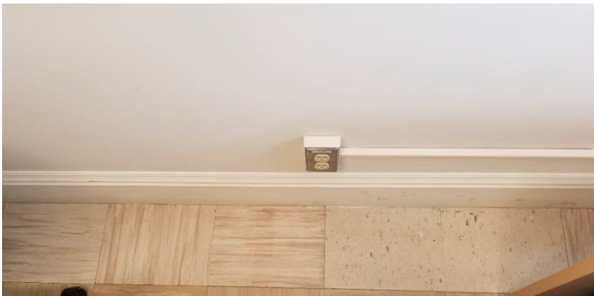
Photo 5: View of asbestos-containing vinyl floor tiles (off-white/beige) observed in the upper left corner in Room 202.
