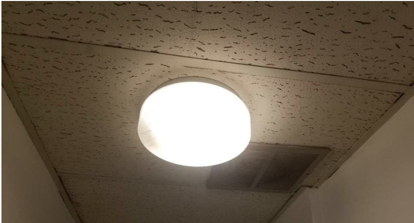
Photo 1: View of asbestos-containing suspended ceiling tiles (pinholes with large fissures) observed in Room 108.
