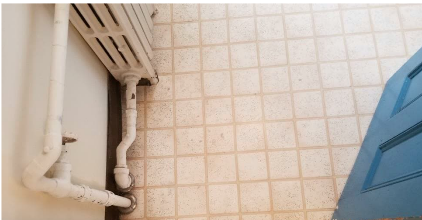
Photo 3: View of previously identified asbestos-containing vinyl sheet flooring (tan squares) observed in Room 209.
