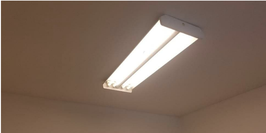
Photo 4: Typical fluorescent light fixtures observed throughout the subject building.
