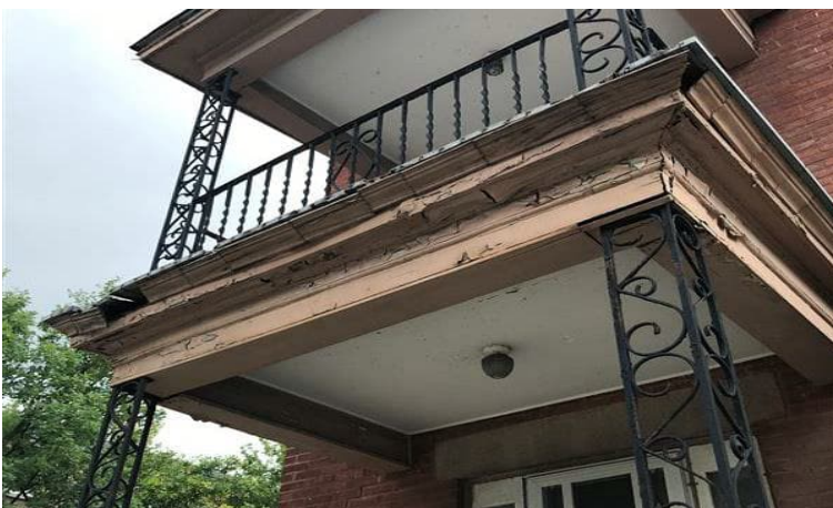
Photo 6: View of lead-containing beige paint observed to be in poor condition on the exterior patio.
