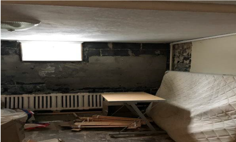
Photo 1: View of typical finishes observed at the building located at 599 King Edward Avenue.
