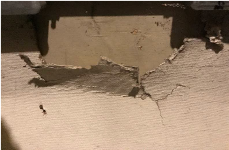
Photo 4: View of asbestos-containing thermal insulation observed to be in poor condition on the wall in the furnace room within the subject building.
