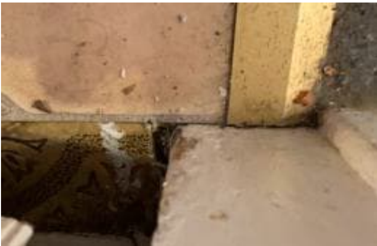
Photo 5: View of asbestos-containing vinyl floor tiles (12"x12"- beige) observed underneath vinyl sheet flooring in the kitchen of Apartment 1 within the subject building.
