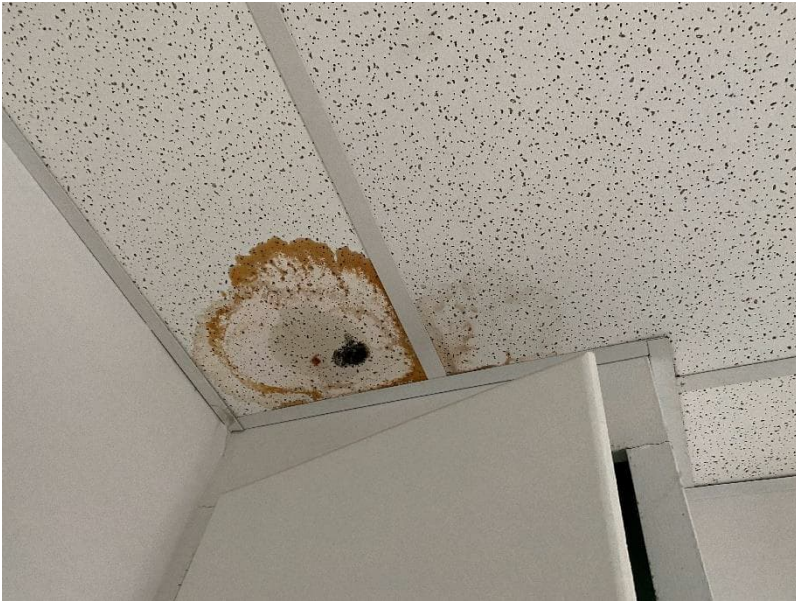
Photo 8: View of water damage observed on ceiling tiles in Room 101 within the subject building during the 2022 Reassessment.
