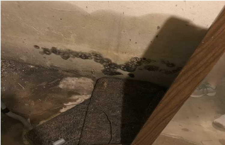
Photo 7: View of mould growth observed in the furnace room within the subject building.
