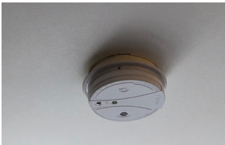
Photo 5: Typical view of smoke detectors containing radioactive materials.
